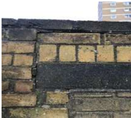
Fig. 8 Cracks in brickwork
