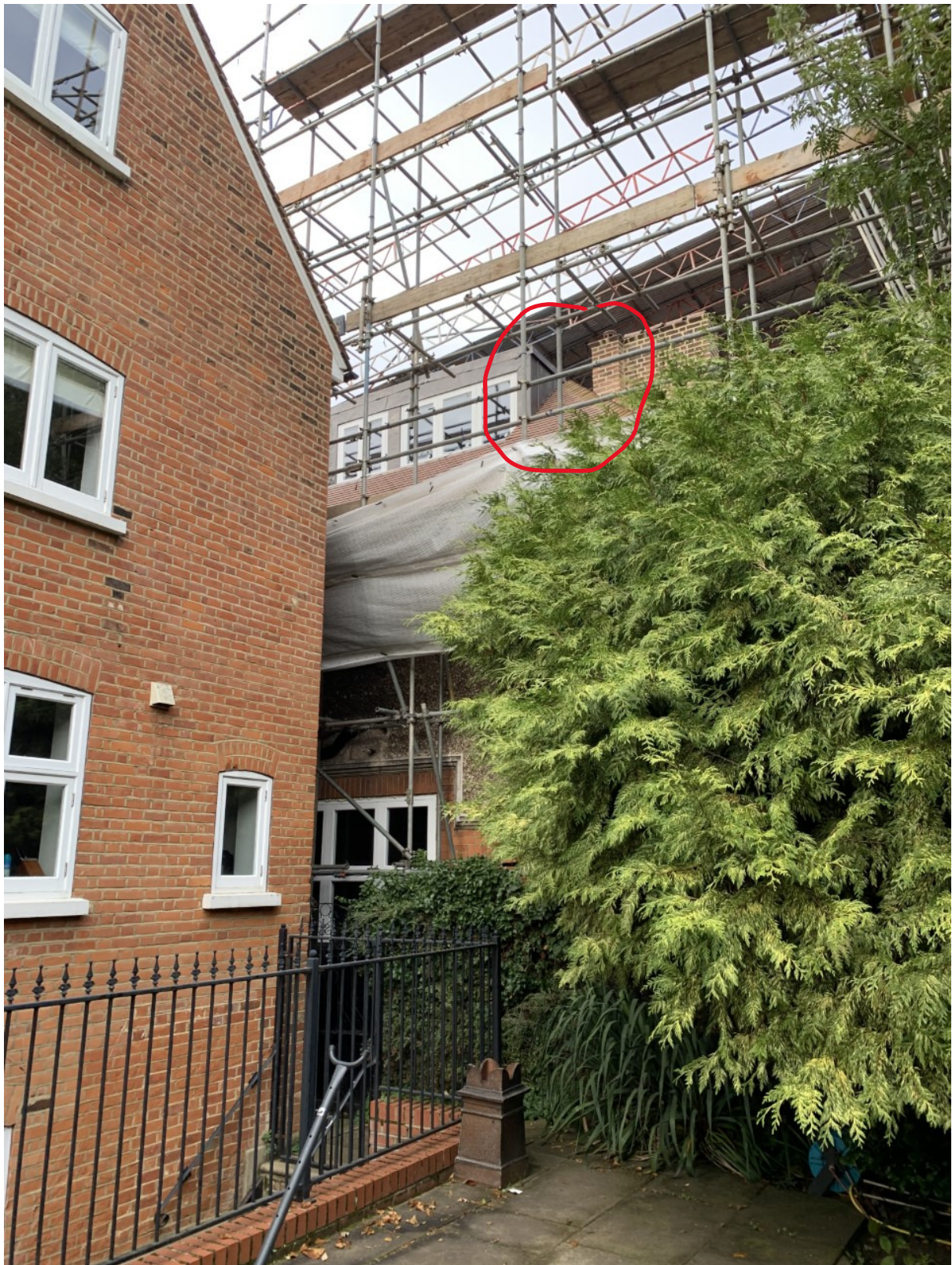
Photo 3 (dormer window after unauthorised works – it is now touching the roof side ridge line and does not have leaded glass windows)
