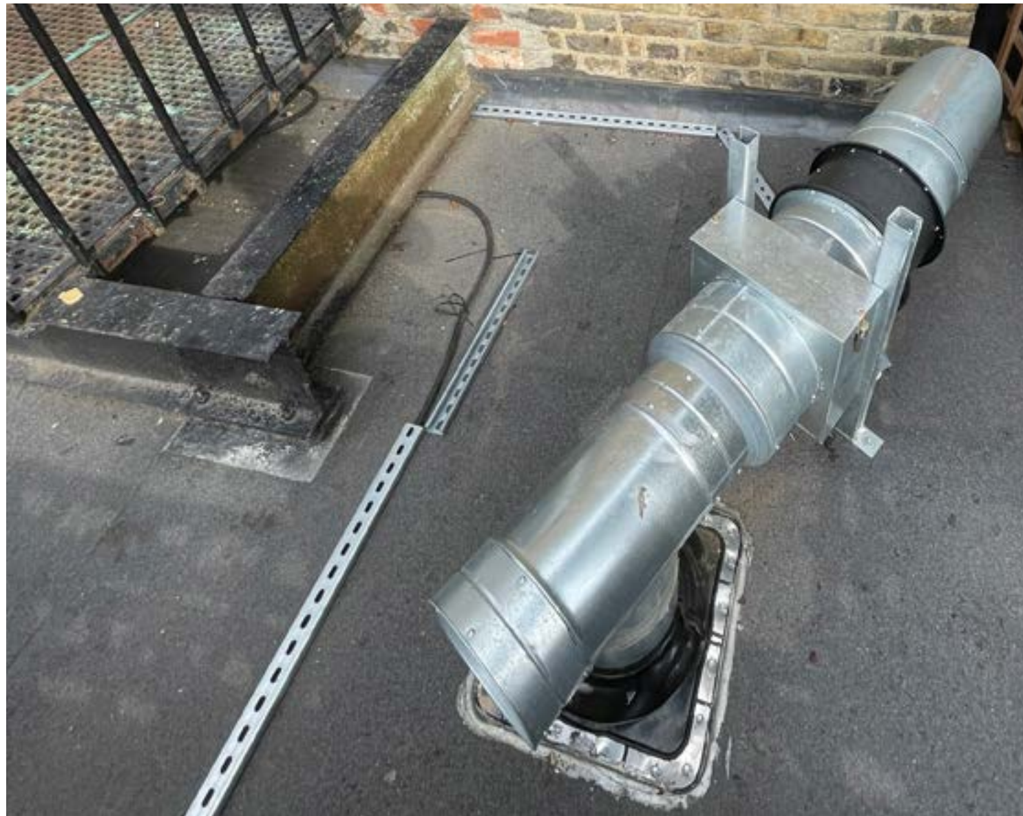
New supply air fan and duct
