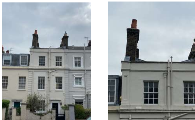
Figure 24 – Showing distorted roof and chimney stack
