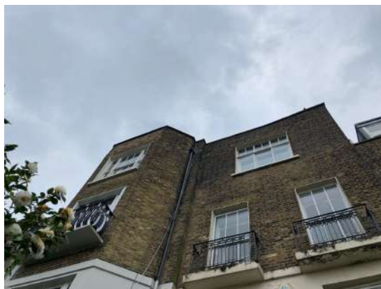
Figure 6. - Showing damaged balconies
