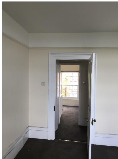
Second floor Deformed Doorway
