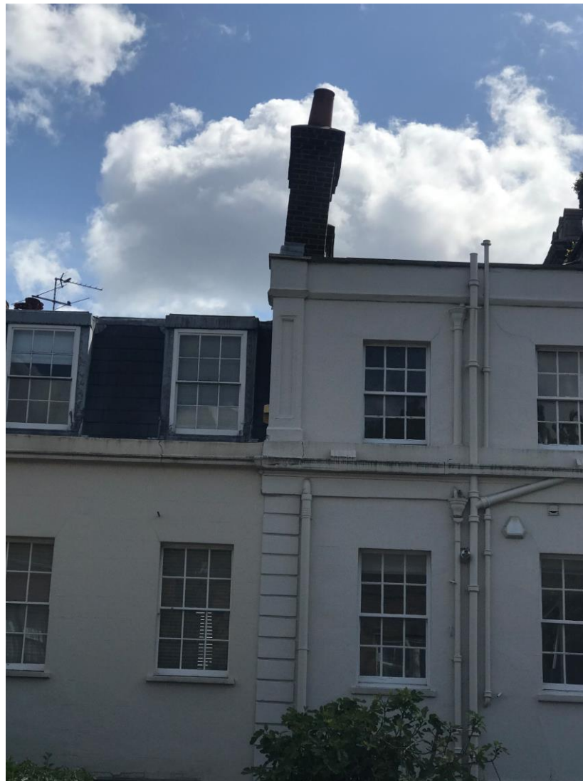
Leaning Chimney Stacks
