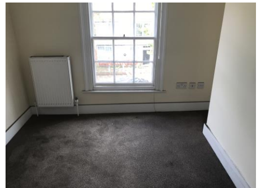
Second Floor Front Room Window Floor Sag Right to Left
