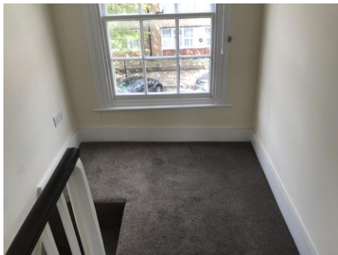
Second Floor Stairway Window Floor Sag Left to Right
