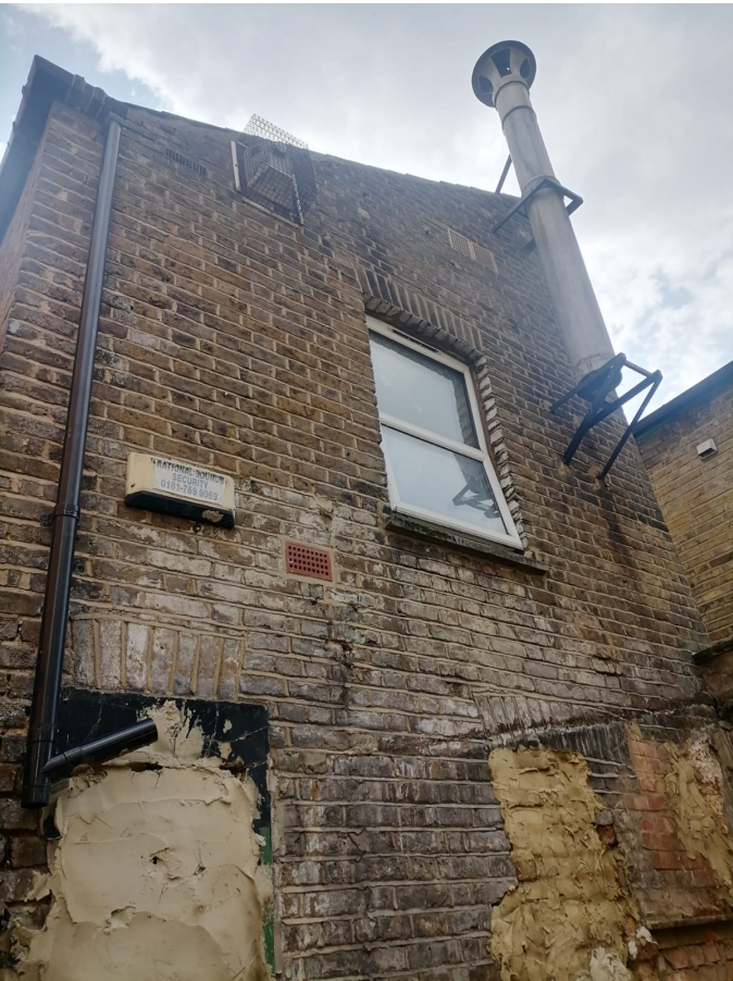
EXISTING VENTILATION PHOTO
