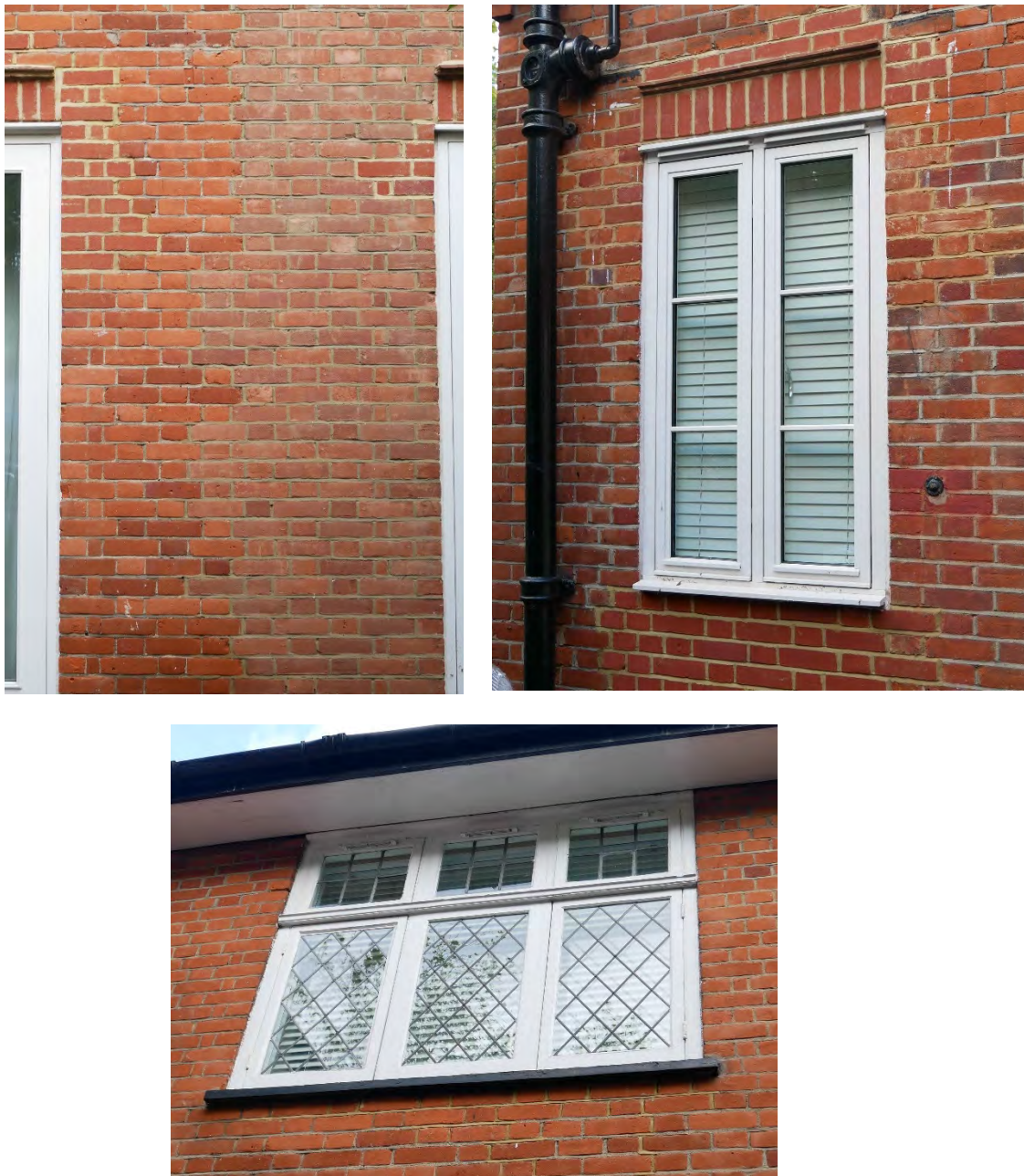
Figure 34: top left; join between later extension and main building, top right; inappropriate windows with UPVC double glazing; bottom; poor quality false leaded lights.
