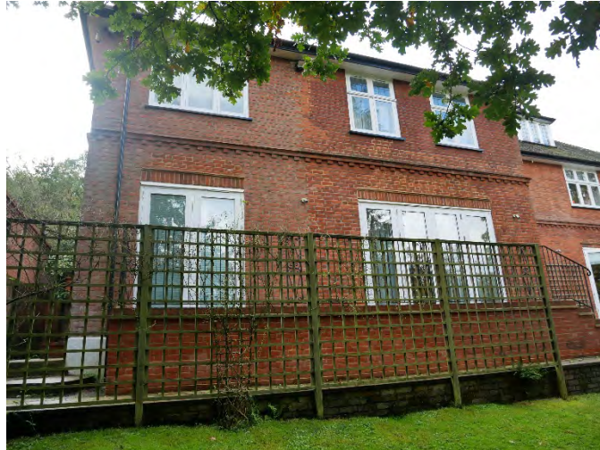
Figure 36: poorly joined extension with different coloured brick and messy pointing
