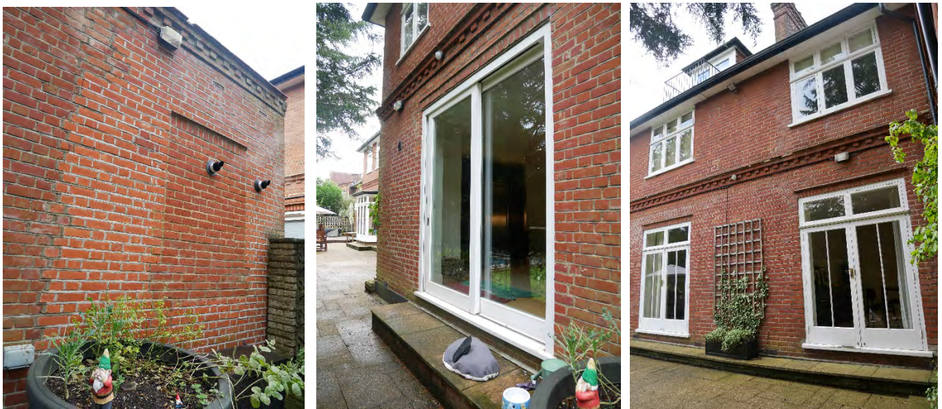
Figure 28: Left, poor choice of brick matching to modern extension; centre, overly large double sliding doors to kitchen; right, fenestration lacking or with inappropriate glazing bars
