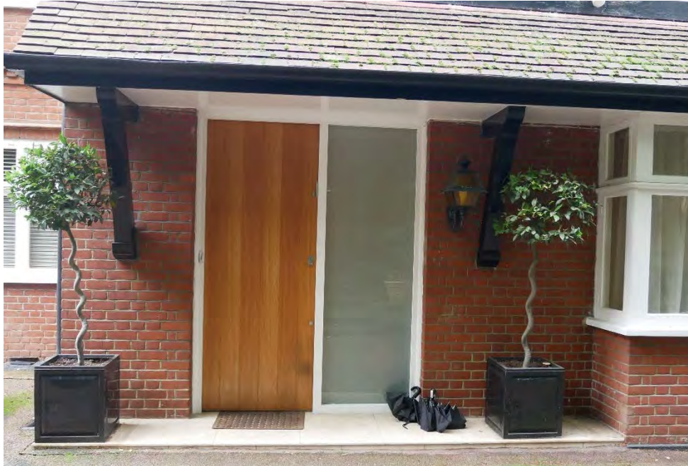
Figure 26: Front door showing replacement door, glass panel and marble doorstep, all inappropriate.
