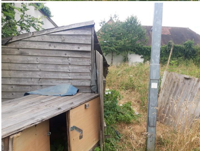
Photograph 2 — Dilapidated shed on site.
