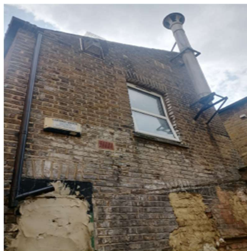
Photo 2. Previous Flue System
