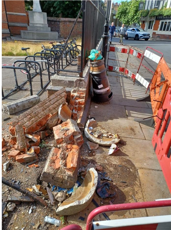
002 – Damaged wall following the vehicle impact
