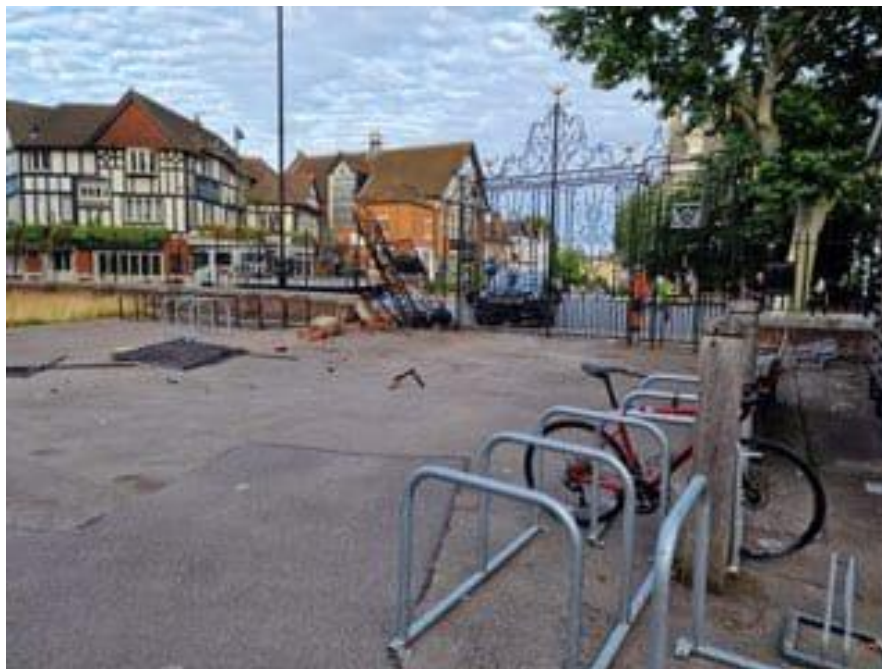
003 – Additional view of the damaged railings
