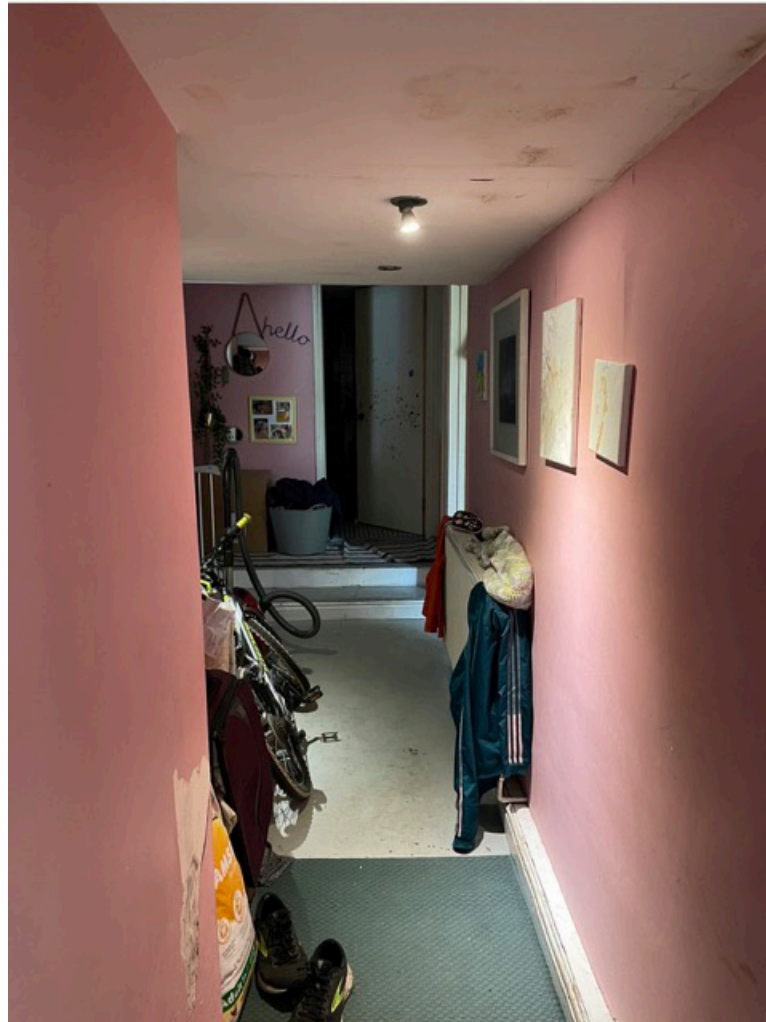
Internal Corridor: The current lower ground flat has low ceilings in the corridor areas, the area is prone to damp and issues of leaking from upstairs flats. The property is in need of organisation
