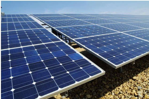
Figure 6: Monocrystalline PV arrays
