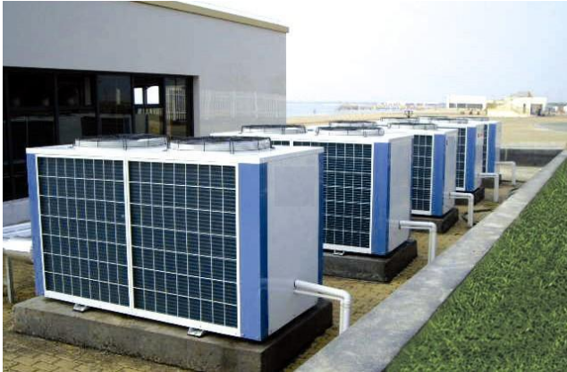
Figure 7: Outdoor units of ASHP
