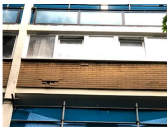
Photograph 1 Loose brick work on east side of building 1. Categorised as providing low potential for roosting bats
