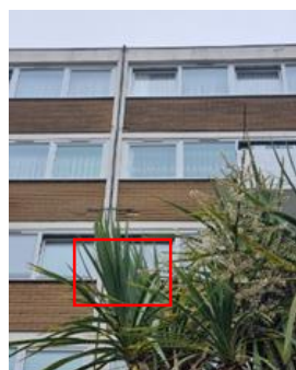
Photograph 6 Damaged brickwork on west side of building 1. (highlighted). Categorised as providing low potential to support roosting bats
