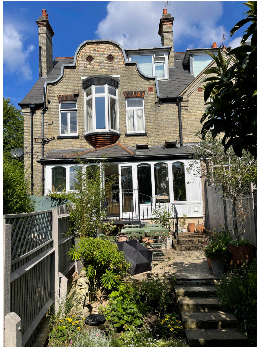
Existing conservatory fenestration does not align to existing windows on levels above.
