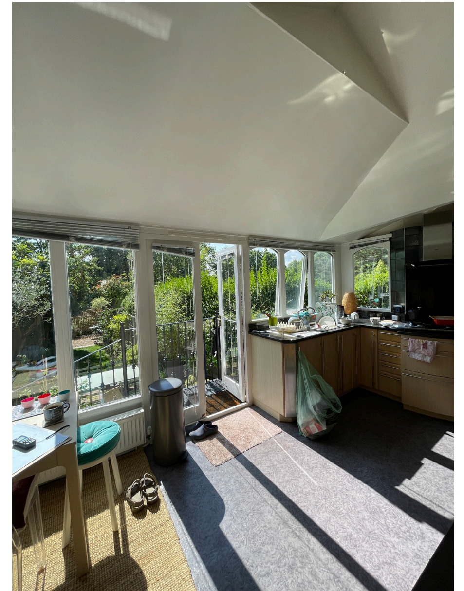
The west-facing wall of the conservatory creates an inefficient internal space due to the multiple-angled facets. The ceiling is awkward due to the strange roof form that is not symmetrical and unsympathetic to the existing building.
