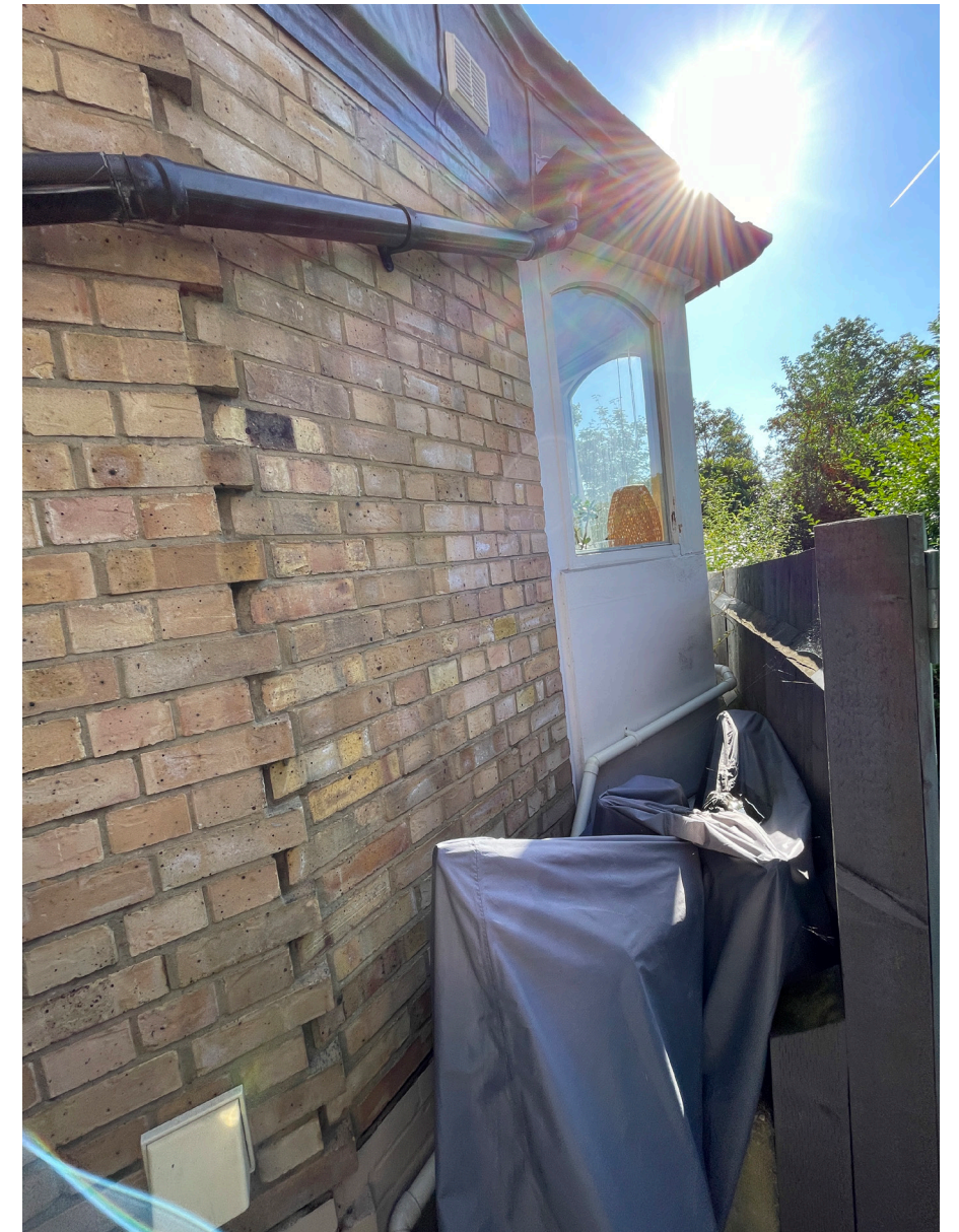
West-facing wall has an awkward form that results in an inefficient space internally.
