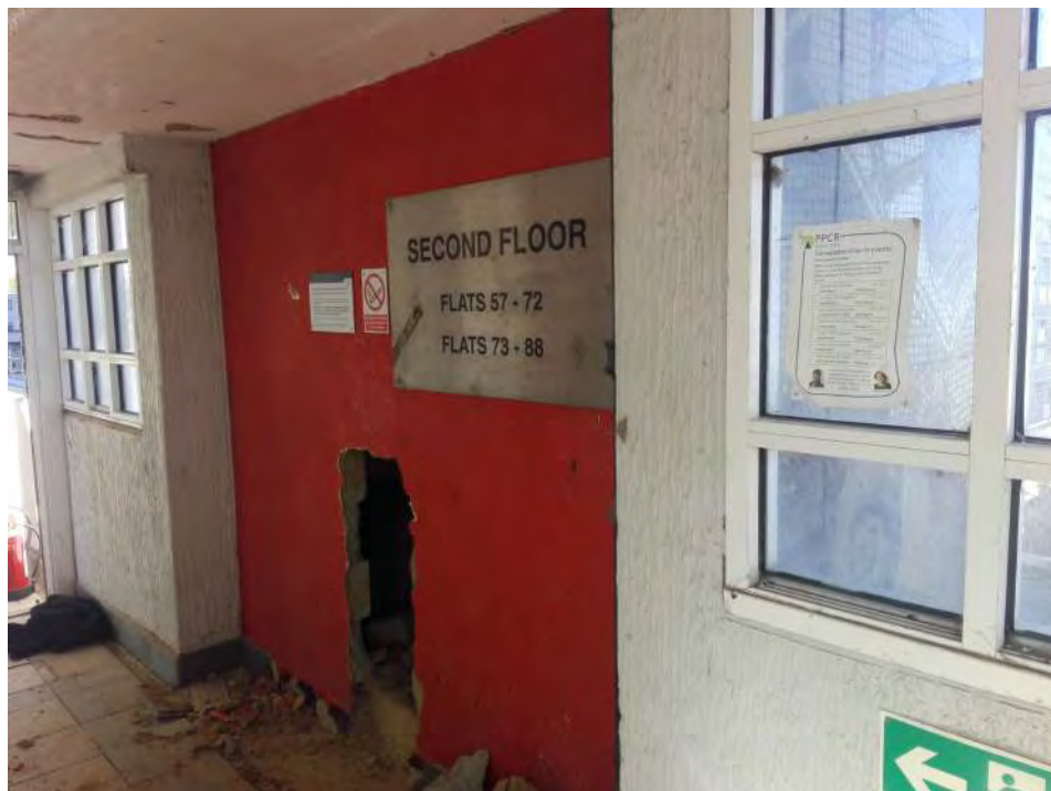
Image 1 - Rubbish chute entrance blocked with a wall
