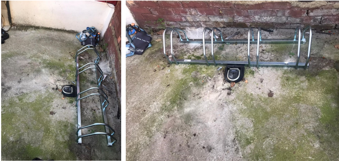
Figure 1: Photographs of installed cycle rack
