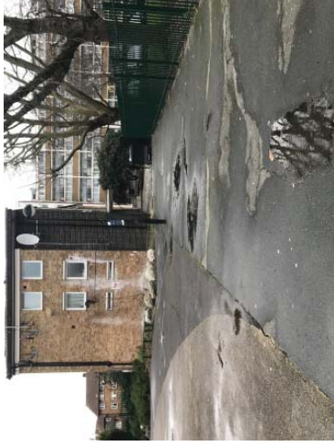
drainage issues within existing play area
