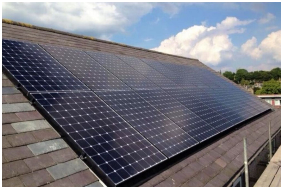
Photovoltaic panels installed on the south facing roof
