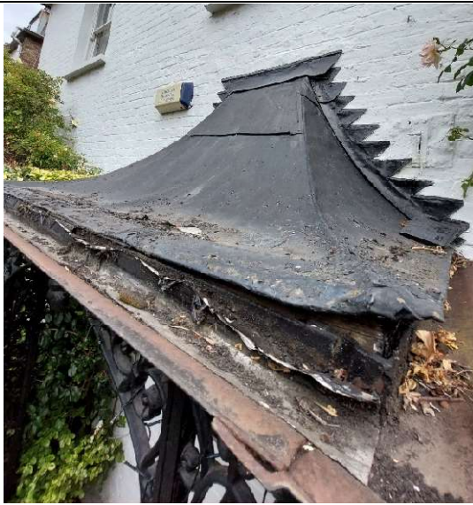
Image 7. Poorly executed temporary flashing repairs to gutter/fascia abutment. Cast Iron gutter in poor condition, joints have failed.
