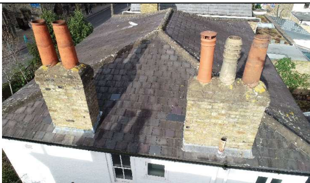
Image 10. Chimneys 1 & 2 Slightly distorted lead detailing. Note: slates have been cut to suit the dimensions of the chimney stack and where tiles are extending off the junction with the flashing, cut tiles have been pieced in rather than using an extended tile (ie. slate and a half) which in turn will lead to movement and potentially water ingress.
