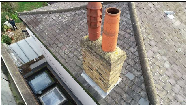
Image 11. Flaunching of Chimney Stack 3 which is cracked and fractured and suffering from algae growth
