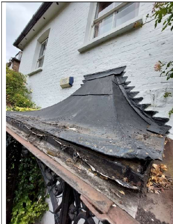
Image 7. Poorly executed temporary flashing repairs to gutter/fascia abutment. Cast Iron gutter in poor condition, joints have failed.
