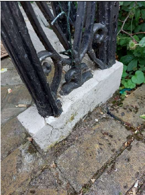
Image 5. Concrete plinths spalling around existing sanctions due to water ingress cause by freeze thaw.
