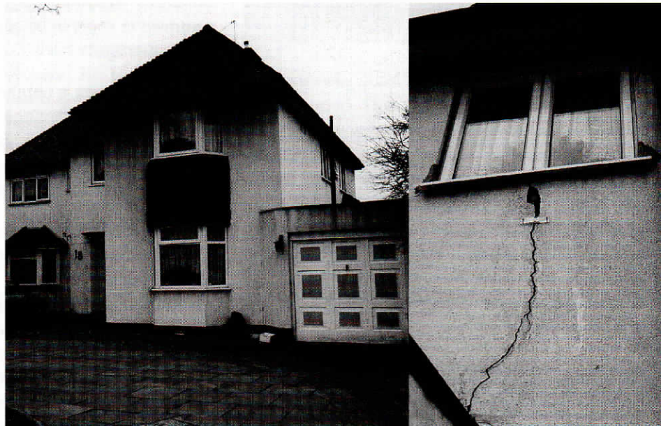
Building with structural cracking
