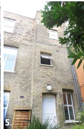
Fig 5: non-cohesive rear facade
