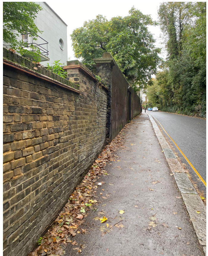
Figure 10 – View from Southwood Lane Looking South showing loose or missing mortar in wall
