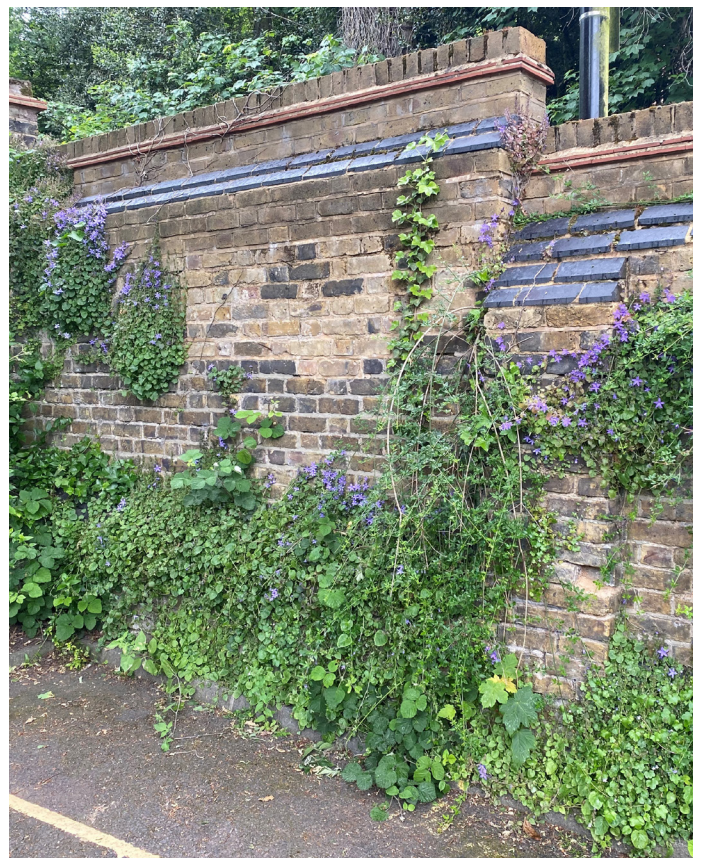
Figure 11 – View from Service road (accessing 86 – 112 Southwood Lane) Looking West showing loose or missing mortar in wall
