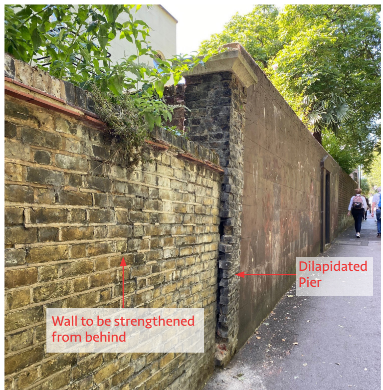
Figure 2- Photograph of the condition of the current Pier and Wall Taken July 2022 showing the extent of deterioration.
