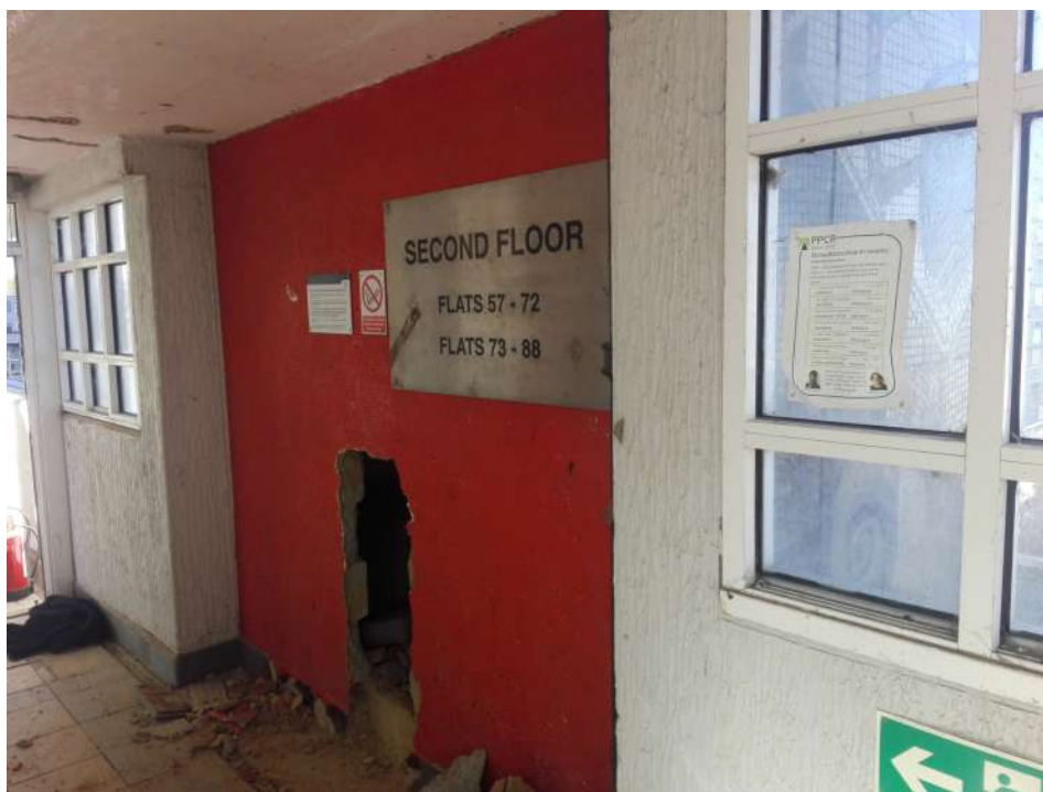
Image 1 - Rubbish chute entrance blocked with a wall
