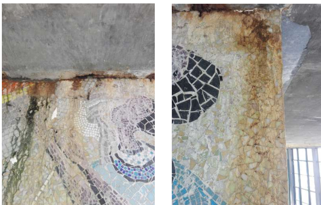
Images 6a-b – Staining caused by rust and saline efflorescences
