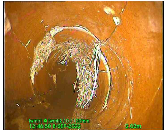
3817.jpg, 00:00:27, 2.05 m Infiltration, dripping at 11 o'clock
