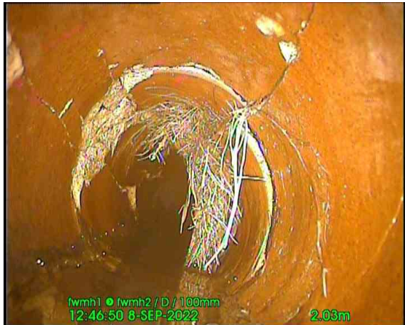
8360.jpg, 00:00:27, 2.05 m Fracture, multiple from 12 o'clock to 12 o'clock
