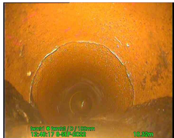
49934.jpg, 00:01:15, 10.32 m Fracture, circumferential from 9 o'clock to 3 o'clock
