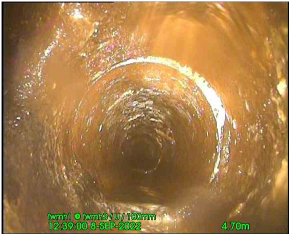
4008.jpg, 00:00:54, 4.70 m Attached deposits, encrustation at joint from 5 o'clock to 7 o'clock, 5% cross-sectional area loss
