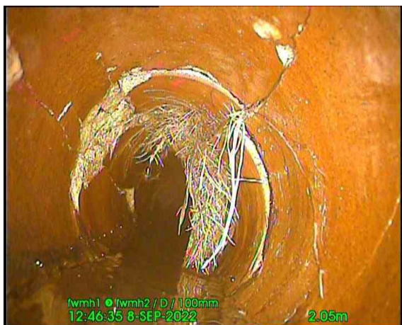
50419.jpg, 00:00:25, 2.05 m Roots, mass, 10% cross-sectional area loss
