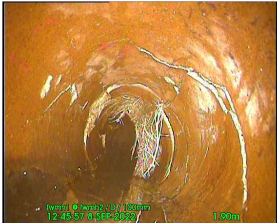
44995.jpg, 00:00:19, 1.90 m Fracture spiral from 11 o'clock to 4 o'clock
