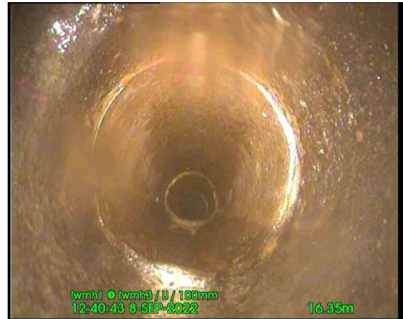
32080.jpg, 00:01:53, 16.35 m Attached deposits, encrustation at joint from 5 o'clock to 7 o'clock, 5% cross-sectional area loss
