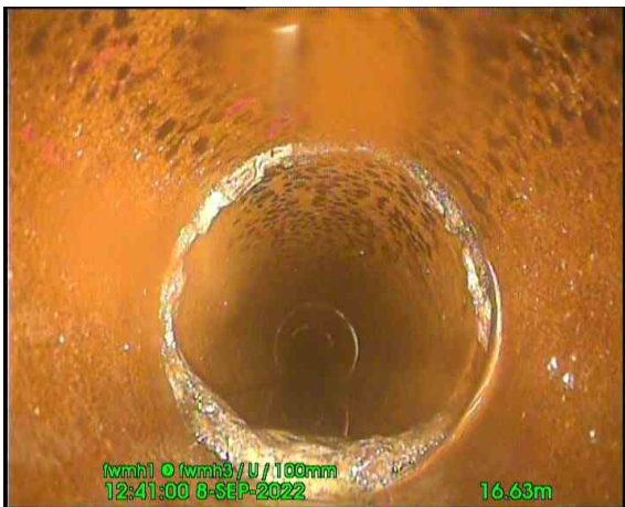
55785.jpg, 00:02:03, 17.02 m Attached deposits, encrustation at joint from 4 o'clock to 8 o'clock, 10% cross-sectional area loss
