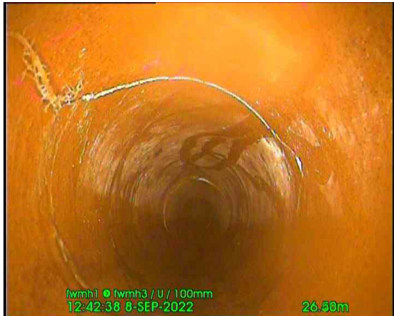
7168.jpg, 00:03:08, 26.58 m Fracture spiral from 10 o'clock to 2 o'clock
