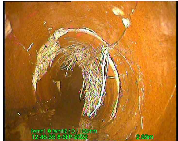
10350.jpg, 00:00:25, 2.05 m Hole in drain or sewer from 9 o'clock to 11 o'clock
