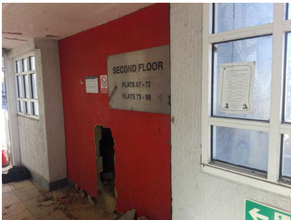
Image 1 - Rubbish chute entrance blocked with a wall
