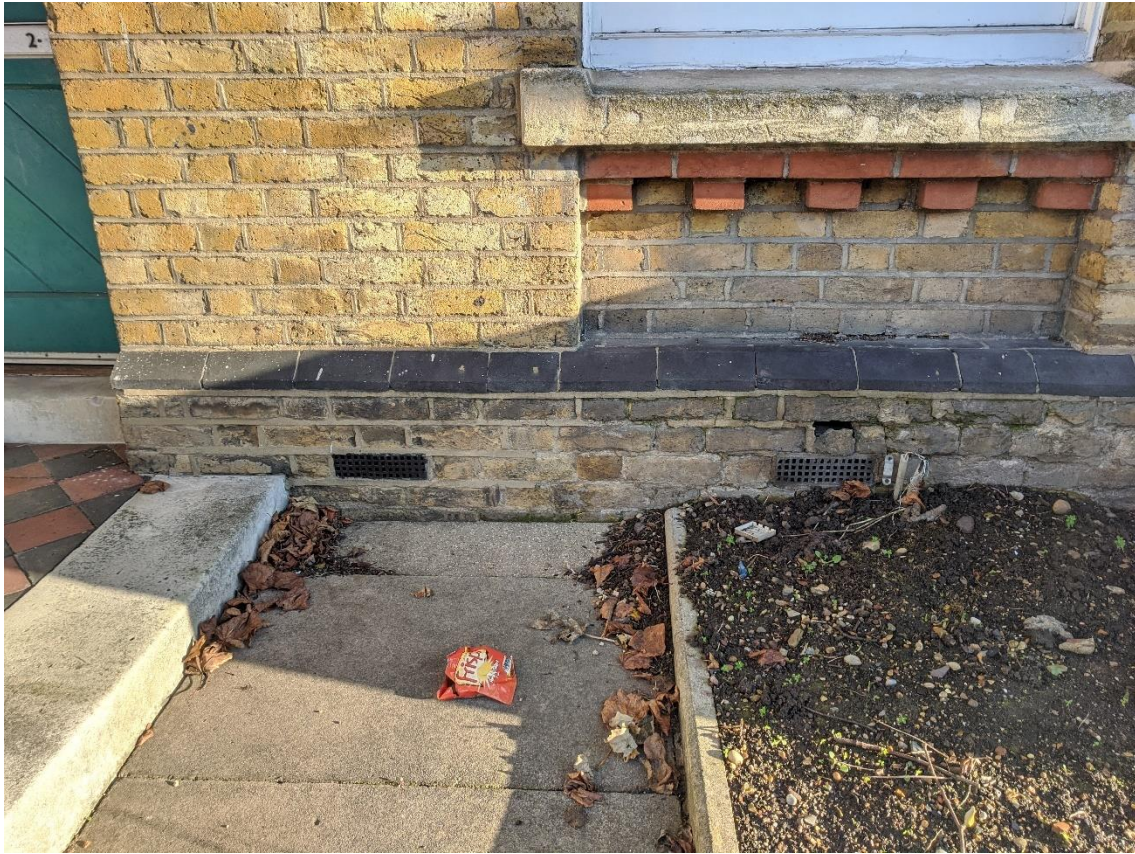
Photograph 3 - Air bricks to Almshouses front elevation
