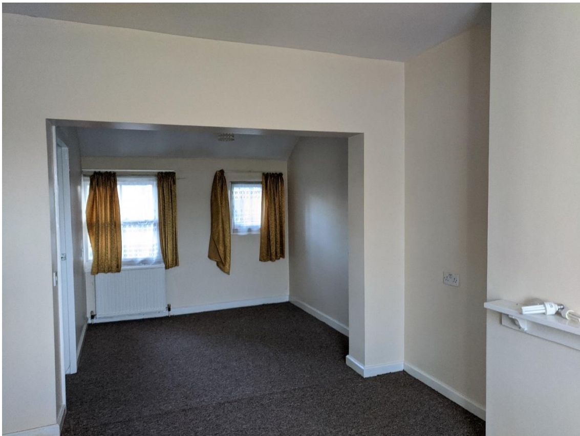
Photograph 6 - Internal condition of ground floor Almshouse (No 25)
