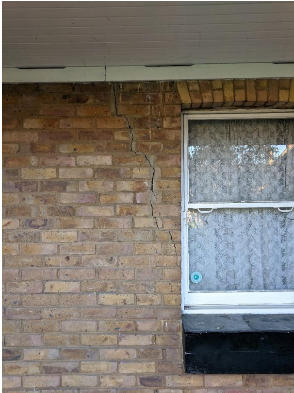
Photograph 11 - Cracking to external wall of 1970's infill block
