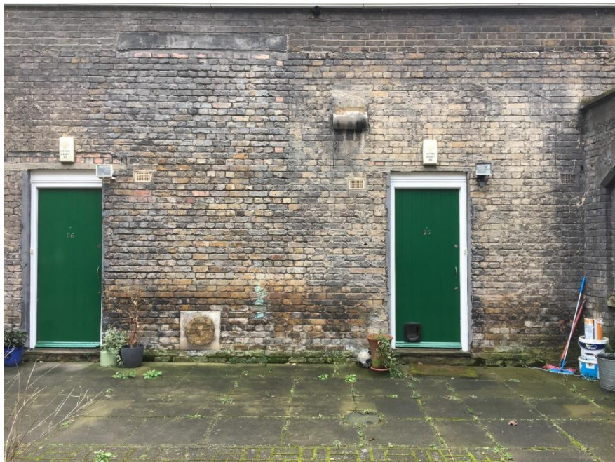
Door to Flat 25 on the right and 26 on the left. Note a) the high level stone corbel that originally supported the roof of a passage, b) the stone head of a former window opening, c) the darkened brickwork (approx. bottom 12 courses) indicating very wet brickwork. Bathrooms are on the opposite side of the wall.
