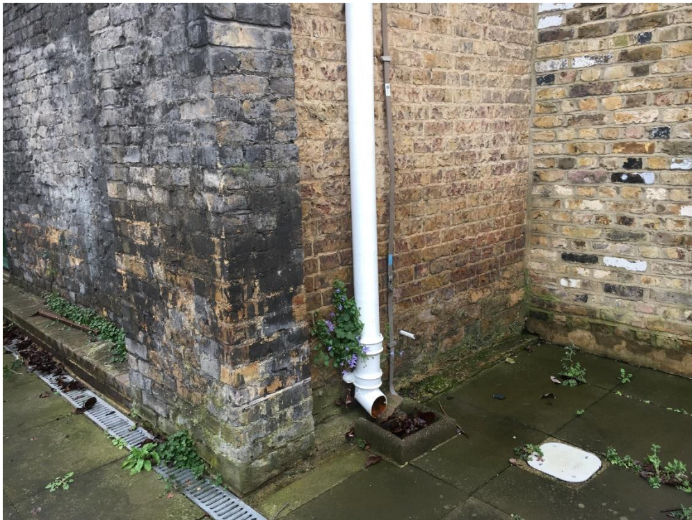
Corner of 24. (The wall that supports the downpipe is the bathroom end wall. The saturation of the wall is marked by the colour change. Also note plant growth. There is no problem with the downpipe.
