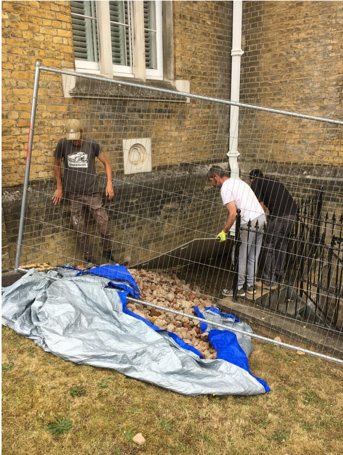
The excavation adjacent to Flat 3 wall. The modern ground level and reset modern drainage gulley are both too high. Both need to be reset to below DPC level.
