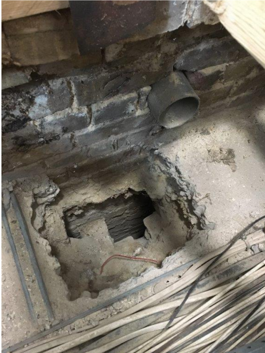
Looking into the corridor underfloor void. The hole in the picture show the breakthrough into the cavity wall construction which is the same as that discovered at the external walls.
