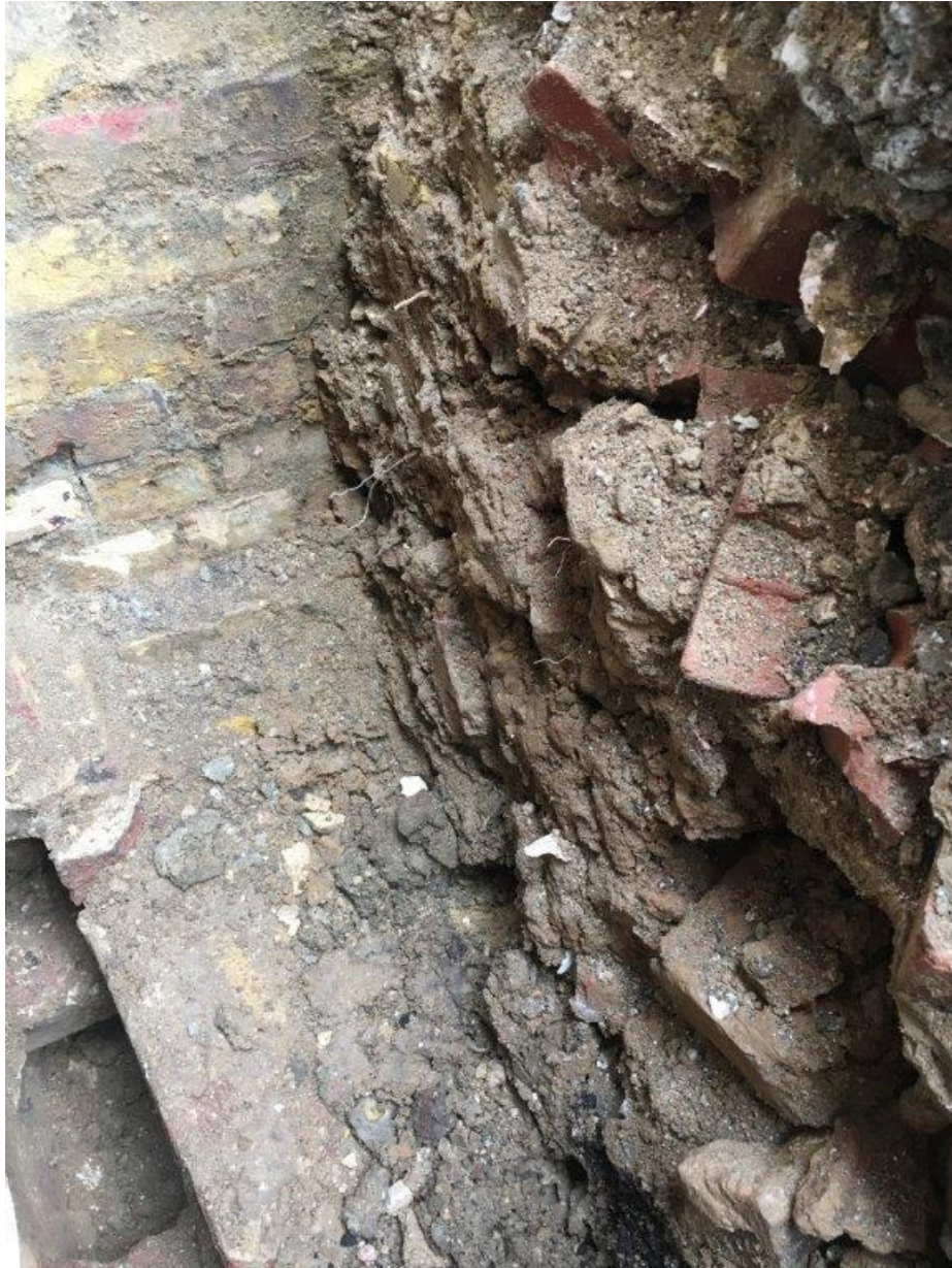
Chaotic backfilling at Pit 1 using it seems demolition material from the school gymnasium and swimming pool buildings.
