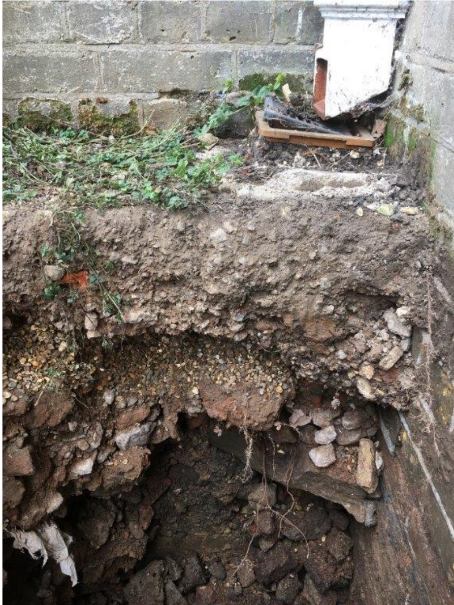
The dig adjacent to the downpipes shows that the existing gulley is inadequate to take the large flow of water from the main roof and it is set above the DPC leading to saturation of the wall. A section of original stone drainage gulley remains in position and is included in this image. It is approx. 10 brick courses below the modern drain, the correct level for finished ground.
