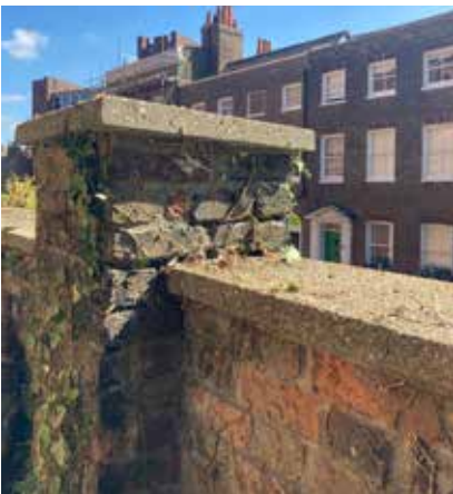
Figure 3.13. Loss of brick face
