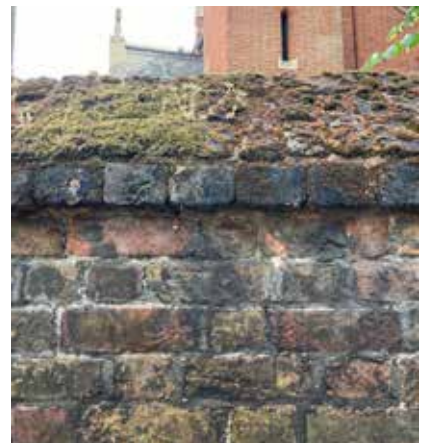
Figure 3.9. Vegetation growth on coping
