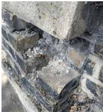
Figure 3.5. Missing bricks beneath coping
