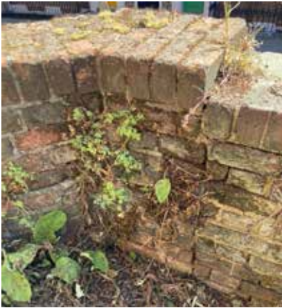
Figure 3.10. Opening joint between brick panels
