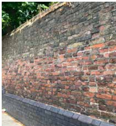
Figure 3.8. Loss of face to High Street elevation
