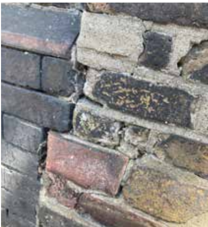
Figure 3.4. Poor jointing between brickwork
