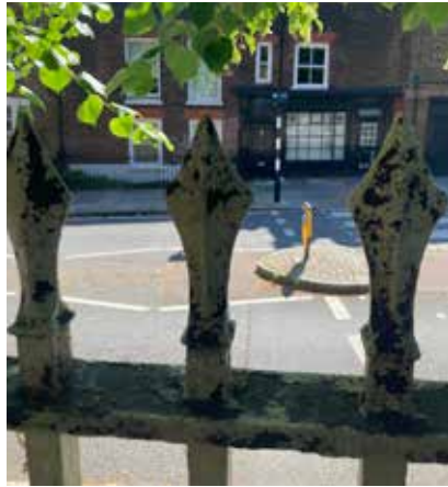
Figure 3.11. Degrading paint finish on railings
