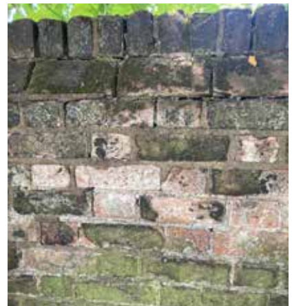
Figure 3.15. Open joints and missing pointing
