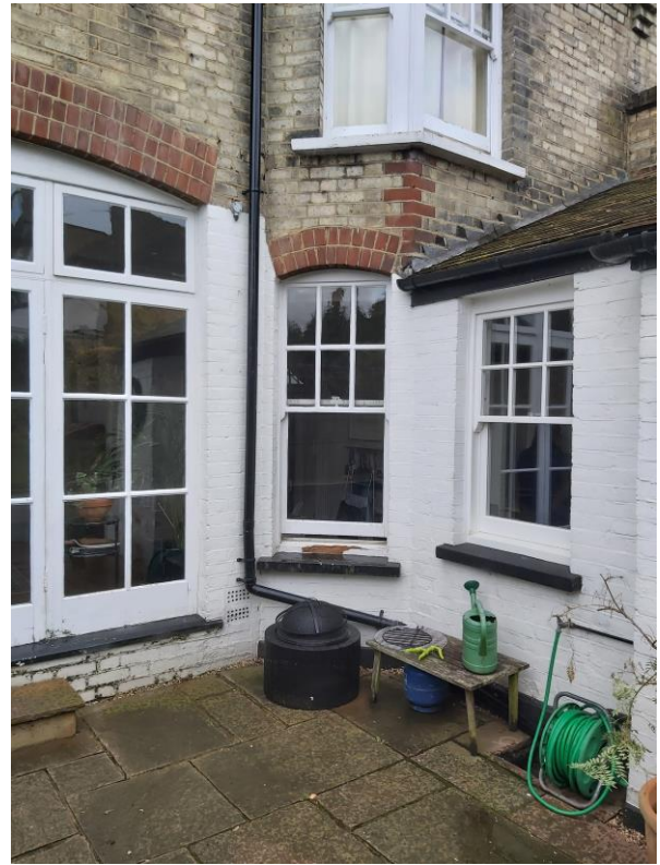
Fig.4 Window to be replaced (centre)
