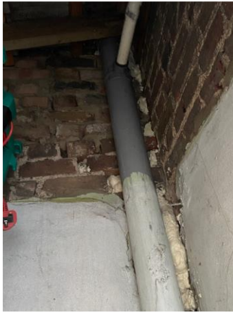
Outhouse wall damage
