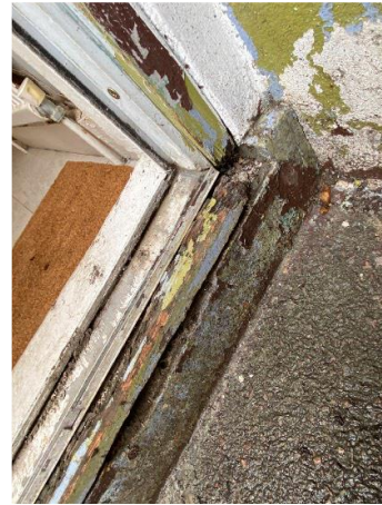
Damage to current door
