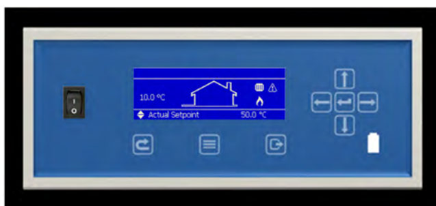
Standard Screenshot of Boiler Controls
