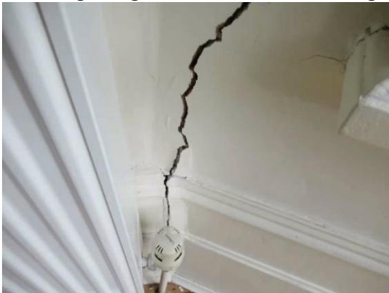
Closed up of Lounge damage.
