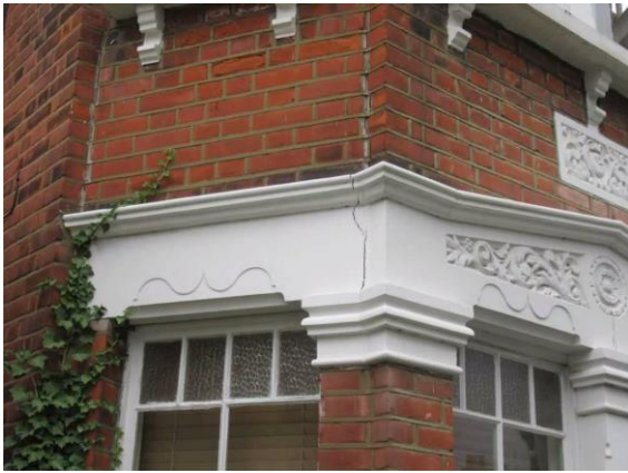
Cracked ornate stonework.
