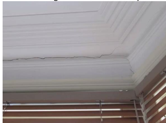
Cracking to ornate coving.
