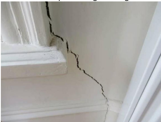
Cracking to the left side of bay.
