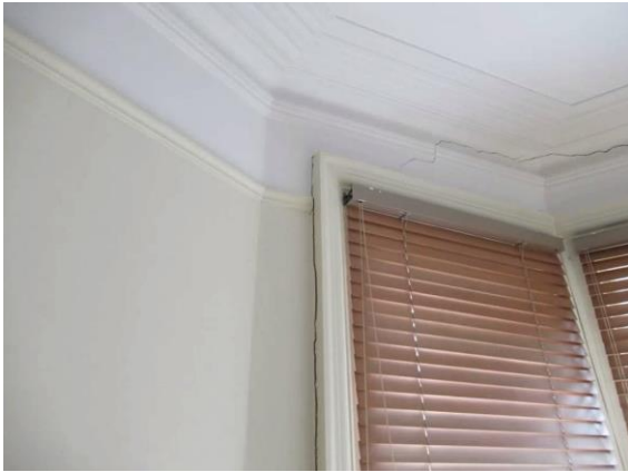
Cracking along window frame and coving.
