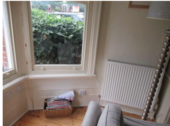
Cracking to the left side of bay.
