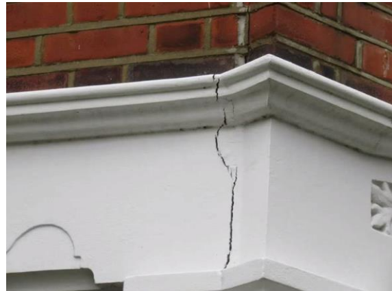
Cracked ornate stonework.
