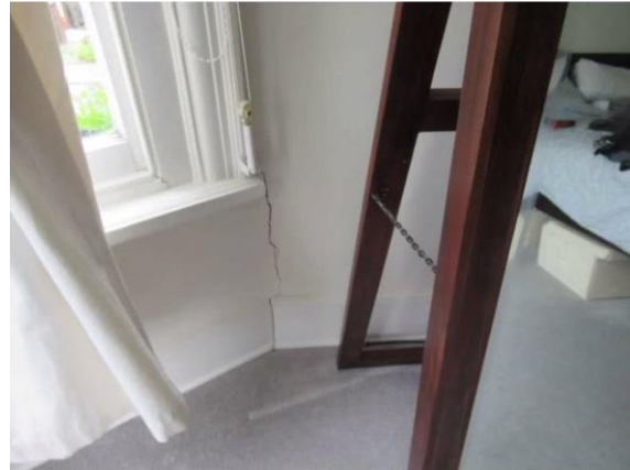
Cracking to left side of bay in Bedroom.
