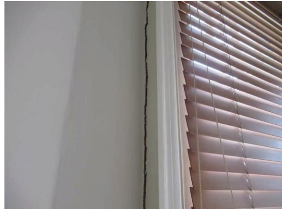
Cracks between woodwork and wall.
