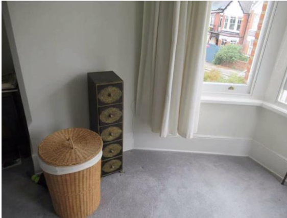
Cracking to bay junction in Bedroom.
