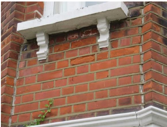
External bay damage.
