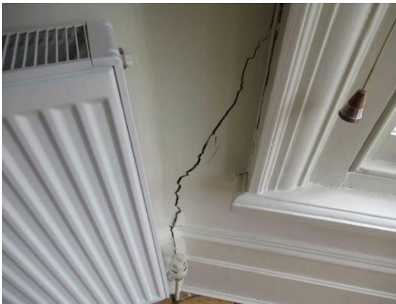
Cracking to right side of bay in Lounge.
