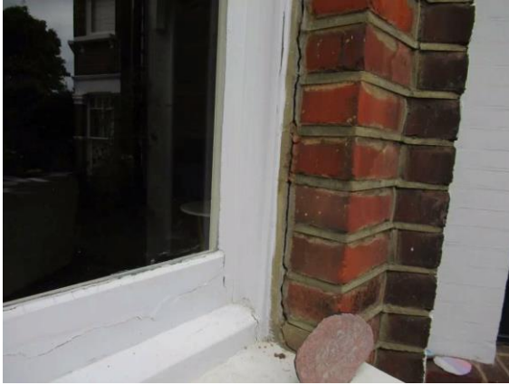
Cracking to mortar on ground floor bay.
