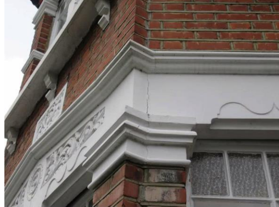
Cracked ornate stonework.
