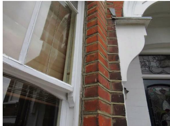
Cracking to mortar.
