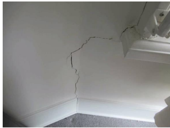
Cracking to bay in Bedroom.
