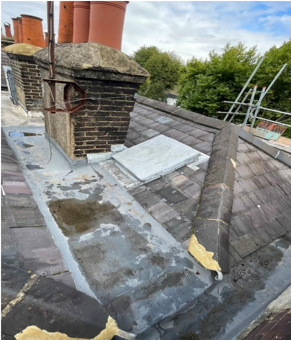
Pic 8) up the central valley showing sunk valley and cement repairs to ridges
