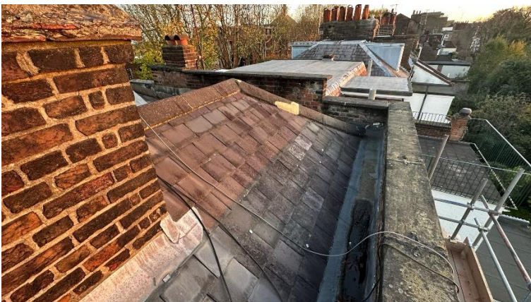
Pic 5) Rear Pitch Valley to hopper has sunk, retaining water
