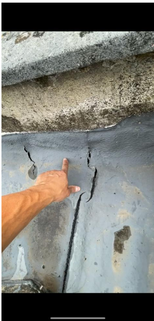
Pic 2) front valley split through mineral and sides are bulging.
