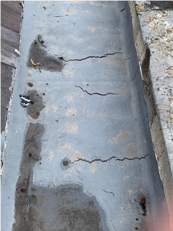
Pic 4) Front valley splits through the liquid covering and deeper than the felt layer
