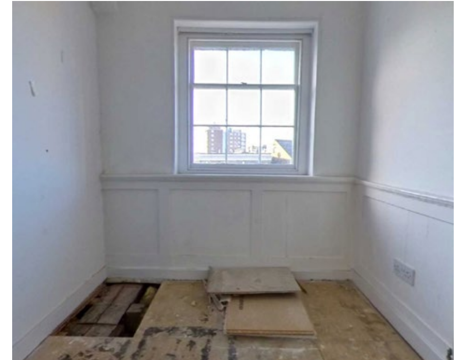
FIGURE 33. 792-S-05 No Evidence Of Floorboards
