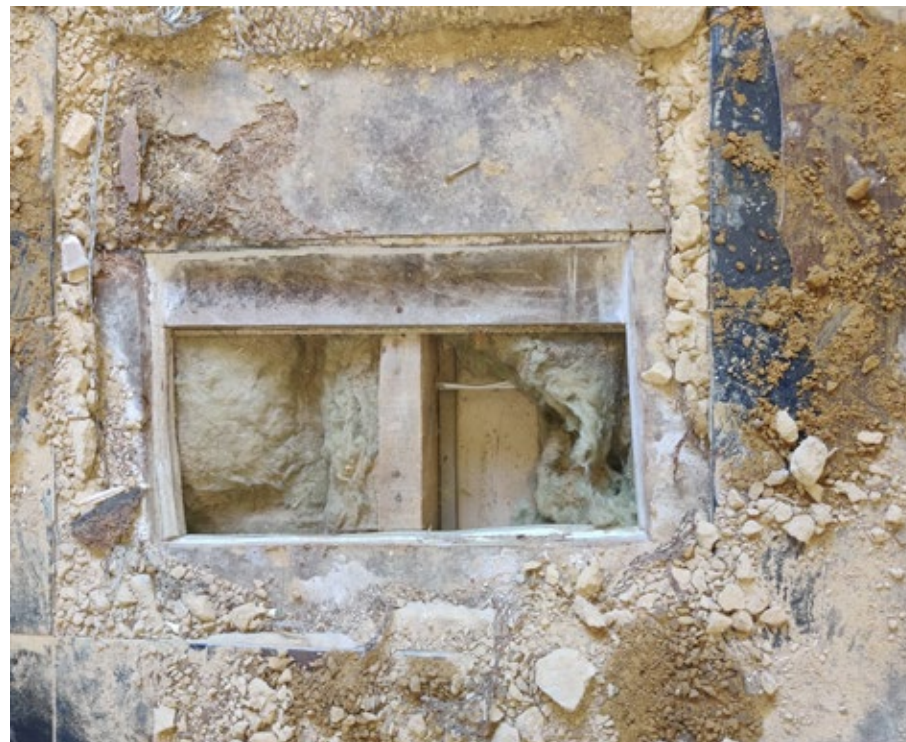
FIGURE 32. 792-S-02 No Evidence Of Floorboards
