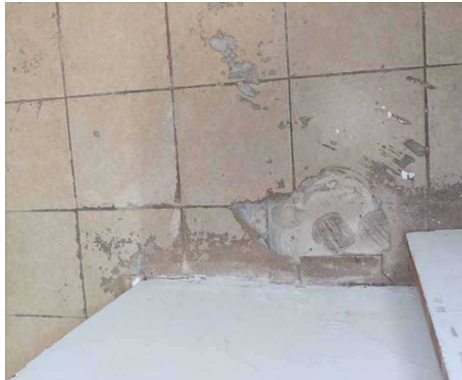
FIGURE 45. No. 792 Server space Rear East
