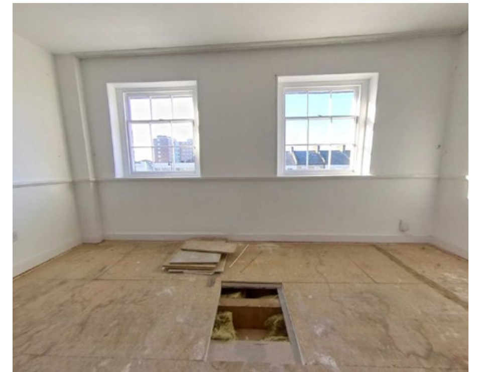
FIGURE 34. 792-S-04 No Evidence Of Floorboards
