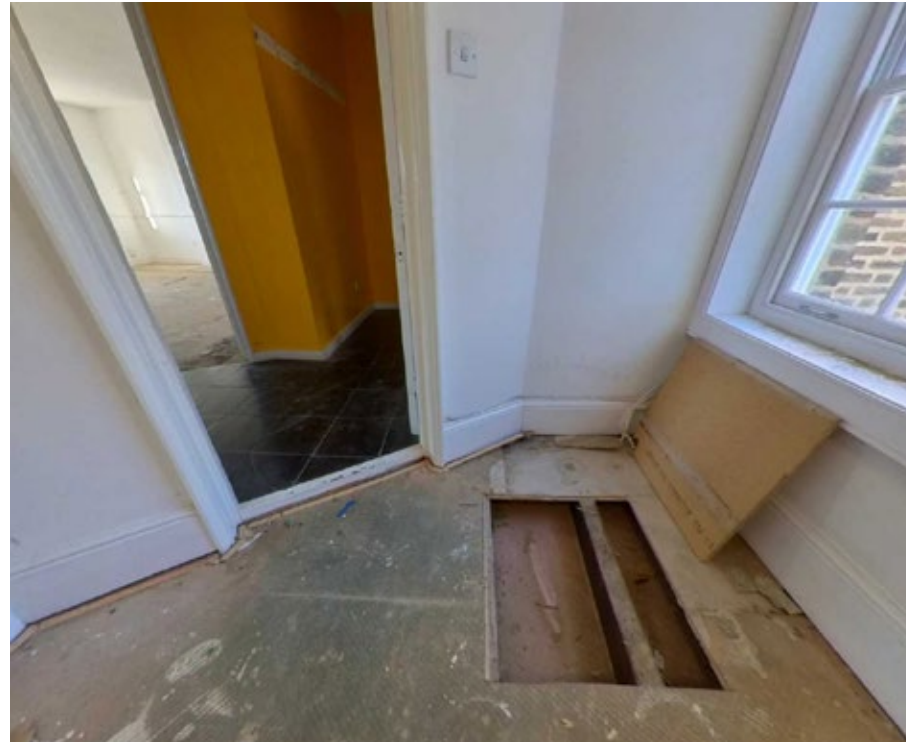
FIGURE 31. 792-S-01 No Evidence Of Floorboards
