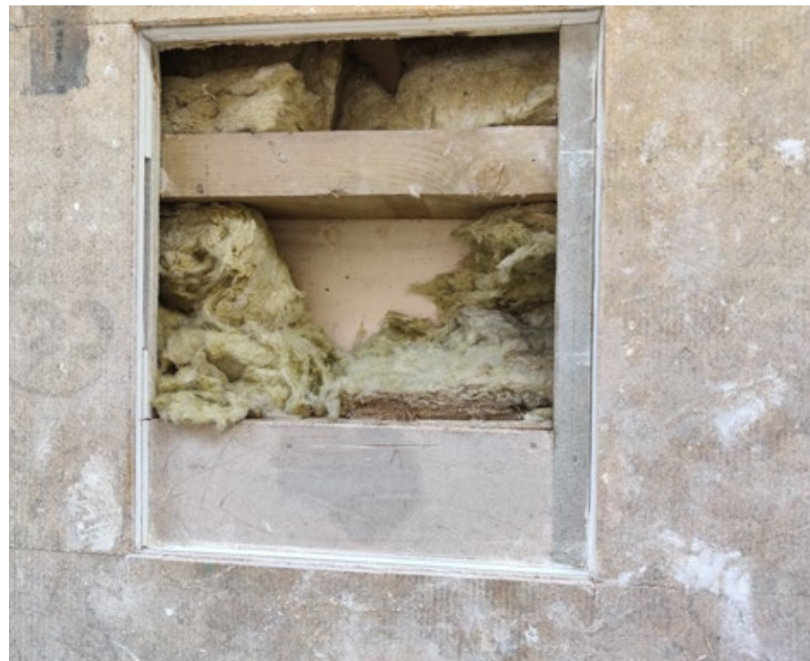
FIGURE 16. 792-G-04 Plasterboard Visible Through The First Floor Room Above
