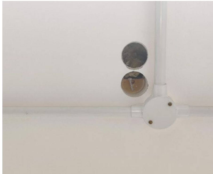
FIGURE 15. 794-B-05 Double Plasterboard Visible Through Investigative Core Hole Within The Ceiling
