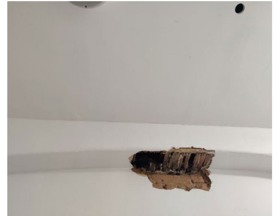
FIGURE 14. Lathe And Plaster Visible Through existing void in the ceiling
