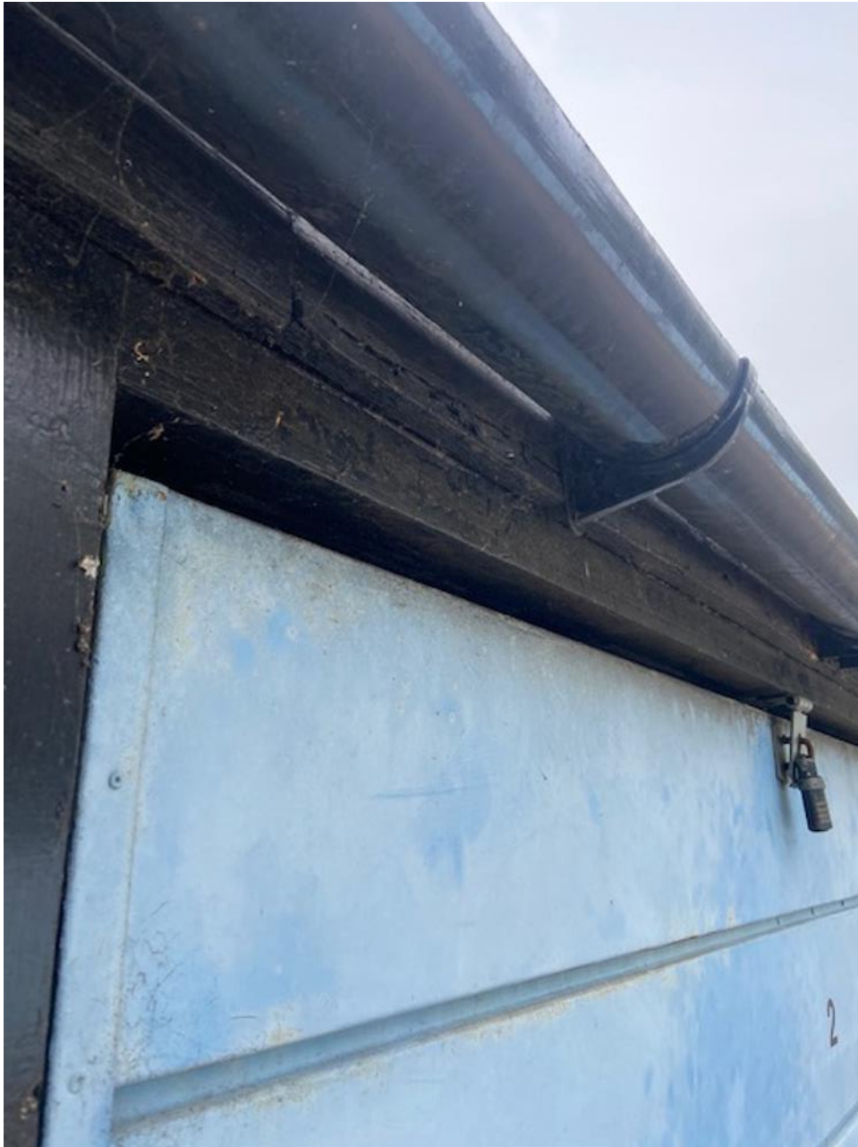
Gap over garage door
