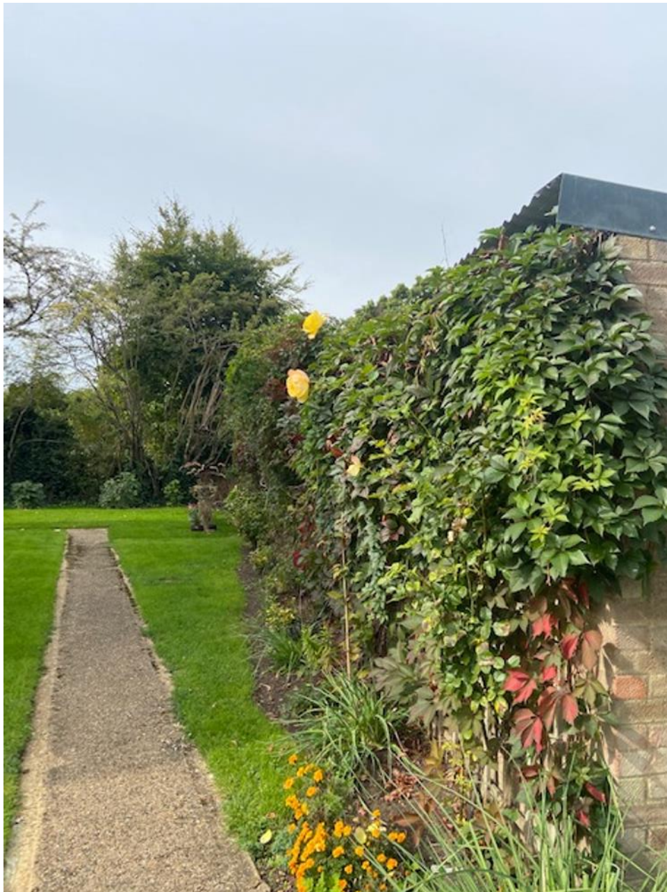
Plant covered rear of southern block of garages
