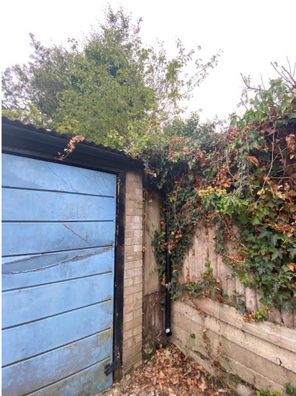
Corner of garages with overgrown vegetation
