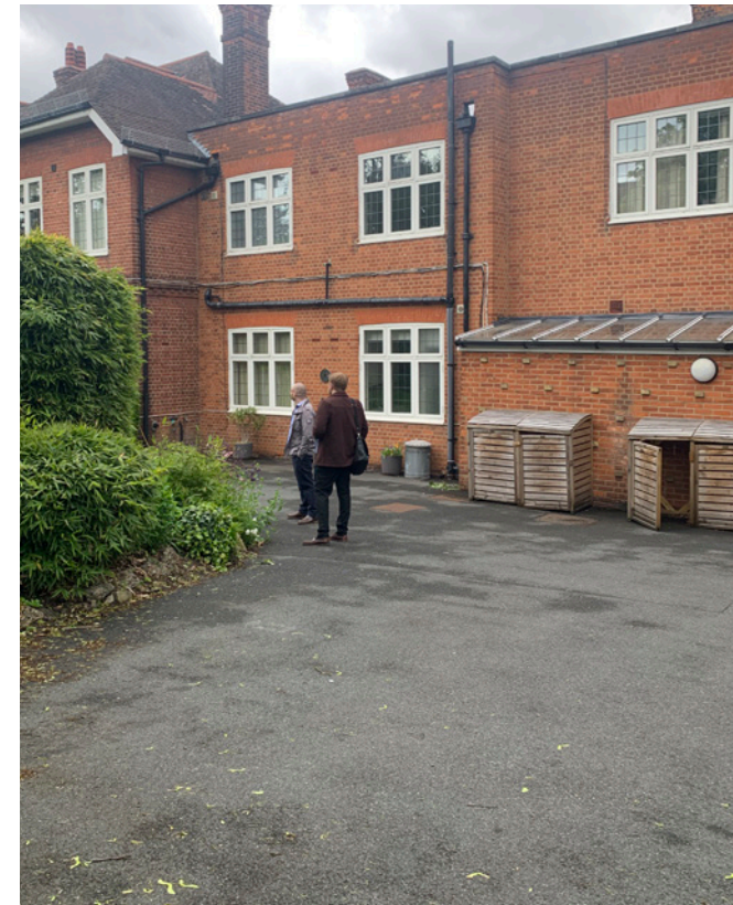
Unsympathetic extension to Kekewich House.
