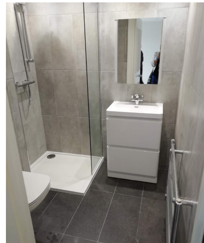
Existing en-suite facilities too small to accommodate staff assistance or wheelchairs
