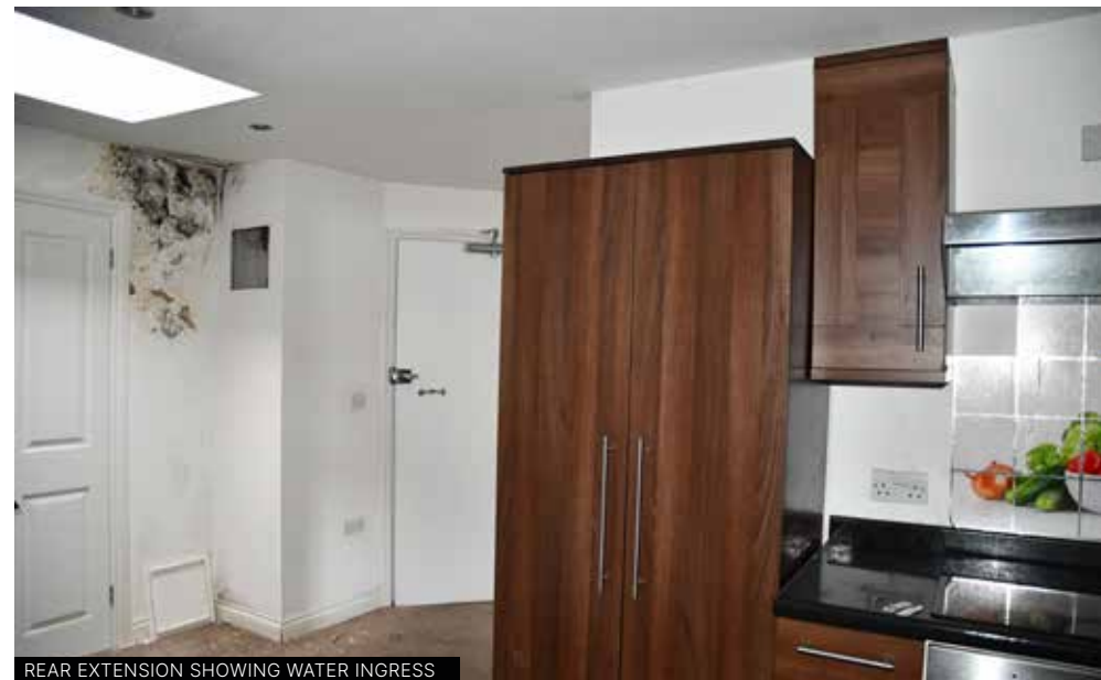
REAR EXTENSION SHOWING WATER INGRESS
