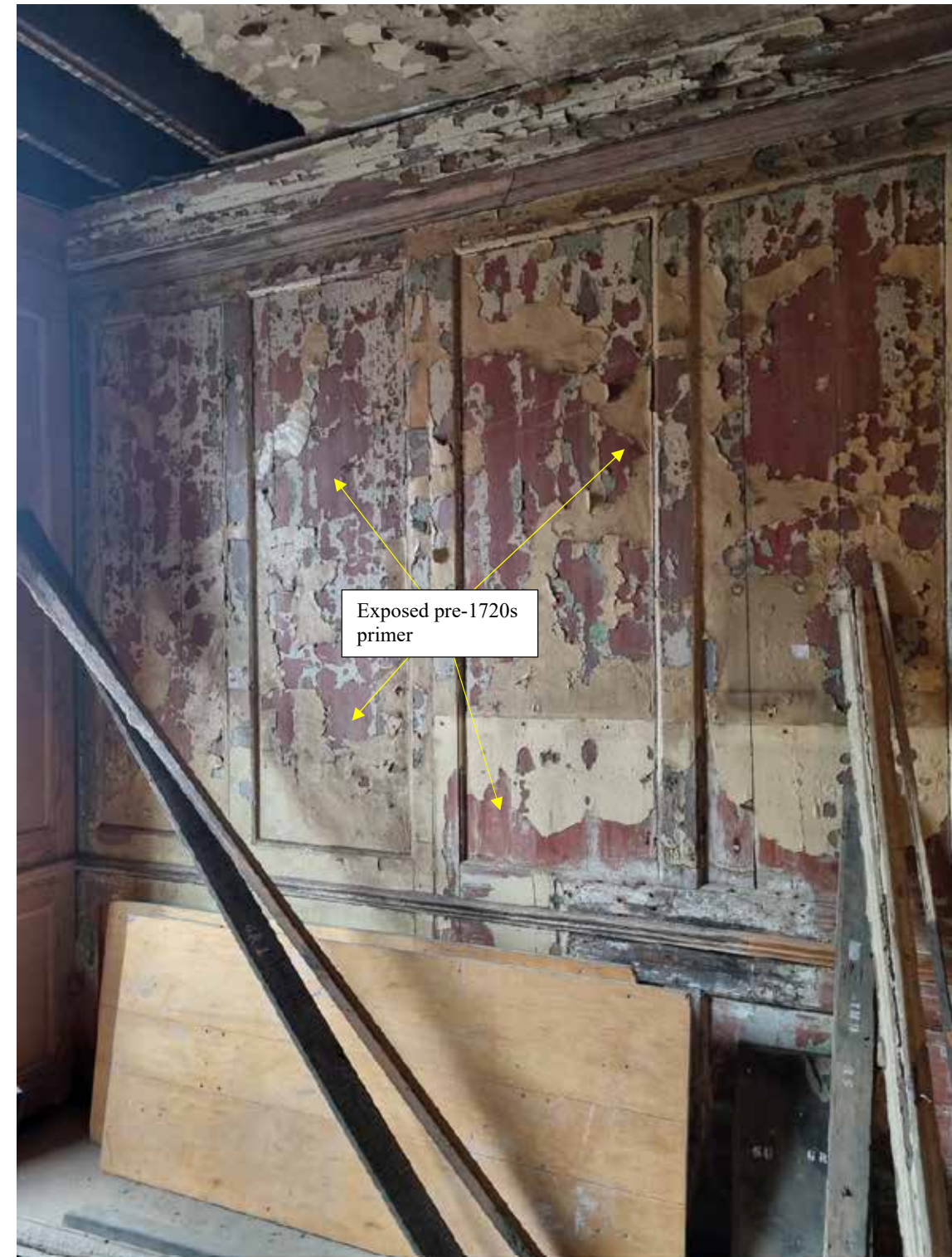
Ground Floor – Front Room. North Wall This shows how the paint has peeled back to the pre-1720s primer
