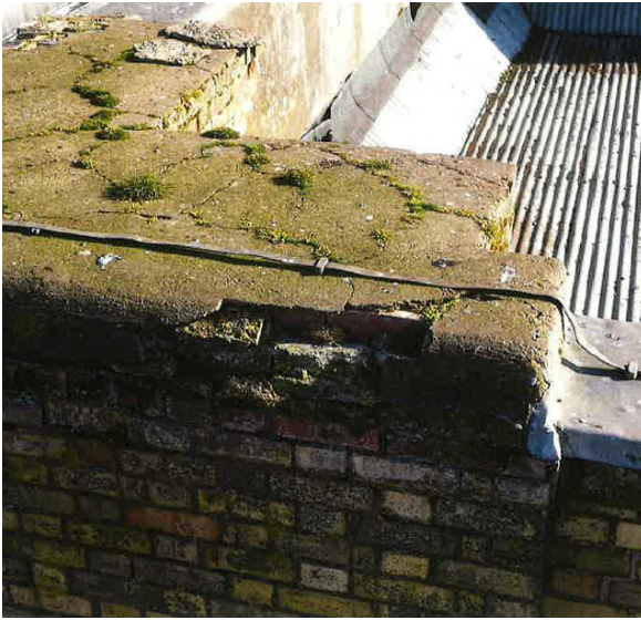
Figure 11: Damage to parapet coping
