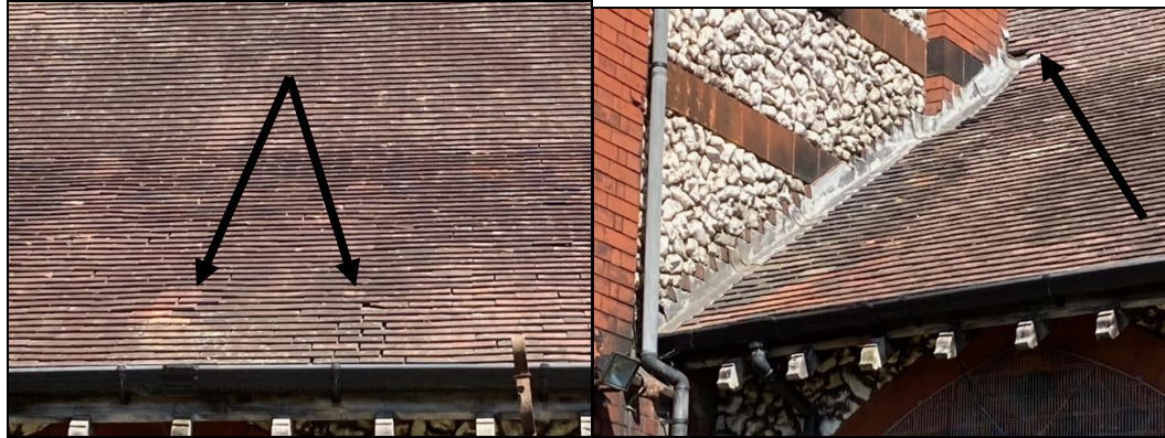
Photographs 7 - 8: Damaged roof tiles & close-fitting valley flashing
