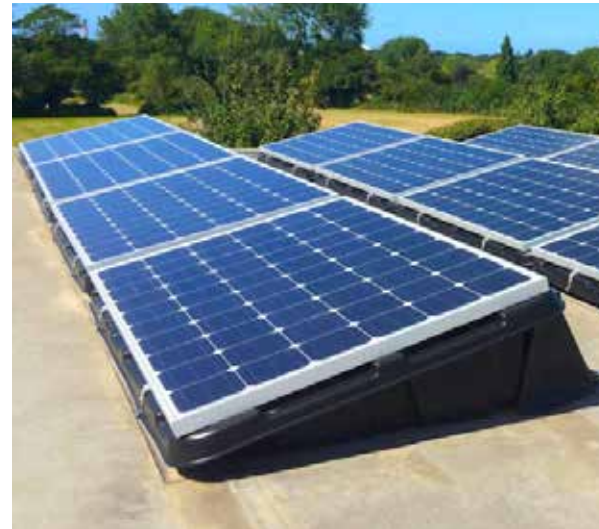
Solar panels on plastic troughs to flat roofs
