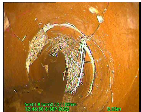
8721.jpg, 00:00:27, 2.05 m Broken pipe from 11 o'clock to 1 o'clock
