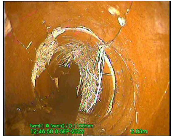
3817.jpg, 00:00:27, 2.05 m Infiltration, dripping at 11 o'clock
