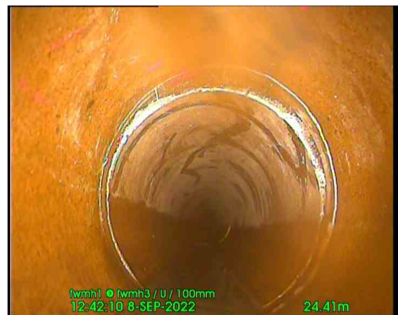
4691.jpg, 00:02:39, 24.41 m Fracture, circumferential at joint from 12 o'clock to 12 o'clock
