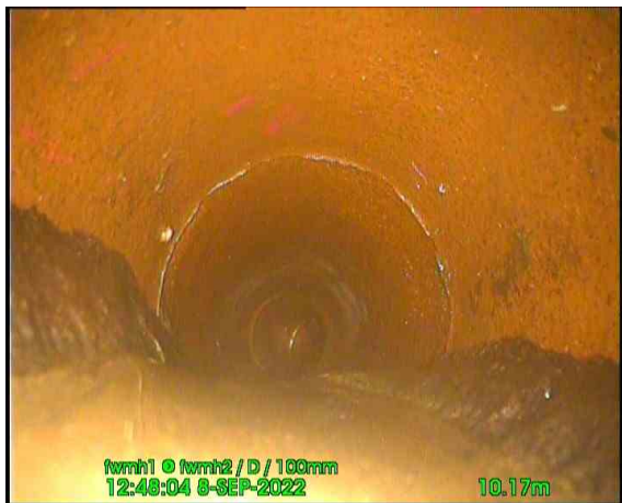
54142.jpg, 00:01:11, 10.17 m Settled deposits, hard or compacted, 30% cross-sectional area loss
