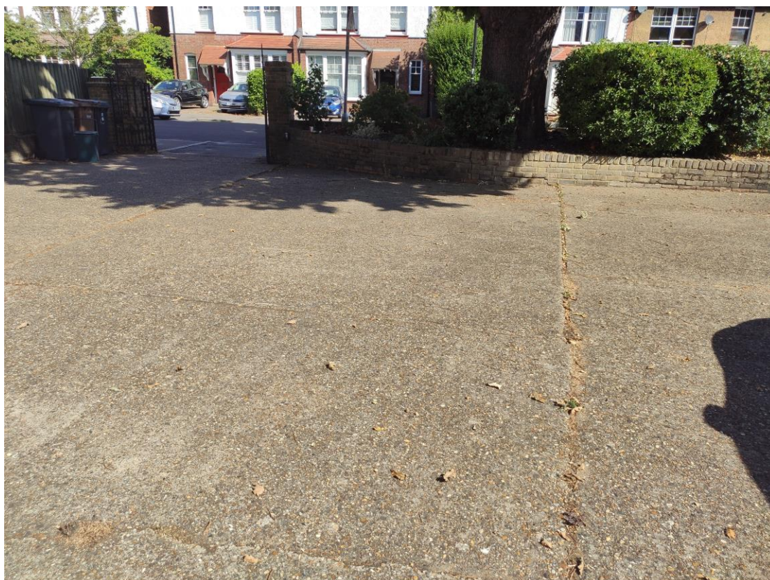
Photograph 5 showing lifting and rotation of concrete drive at 1 St. Martin's Terrace.
