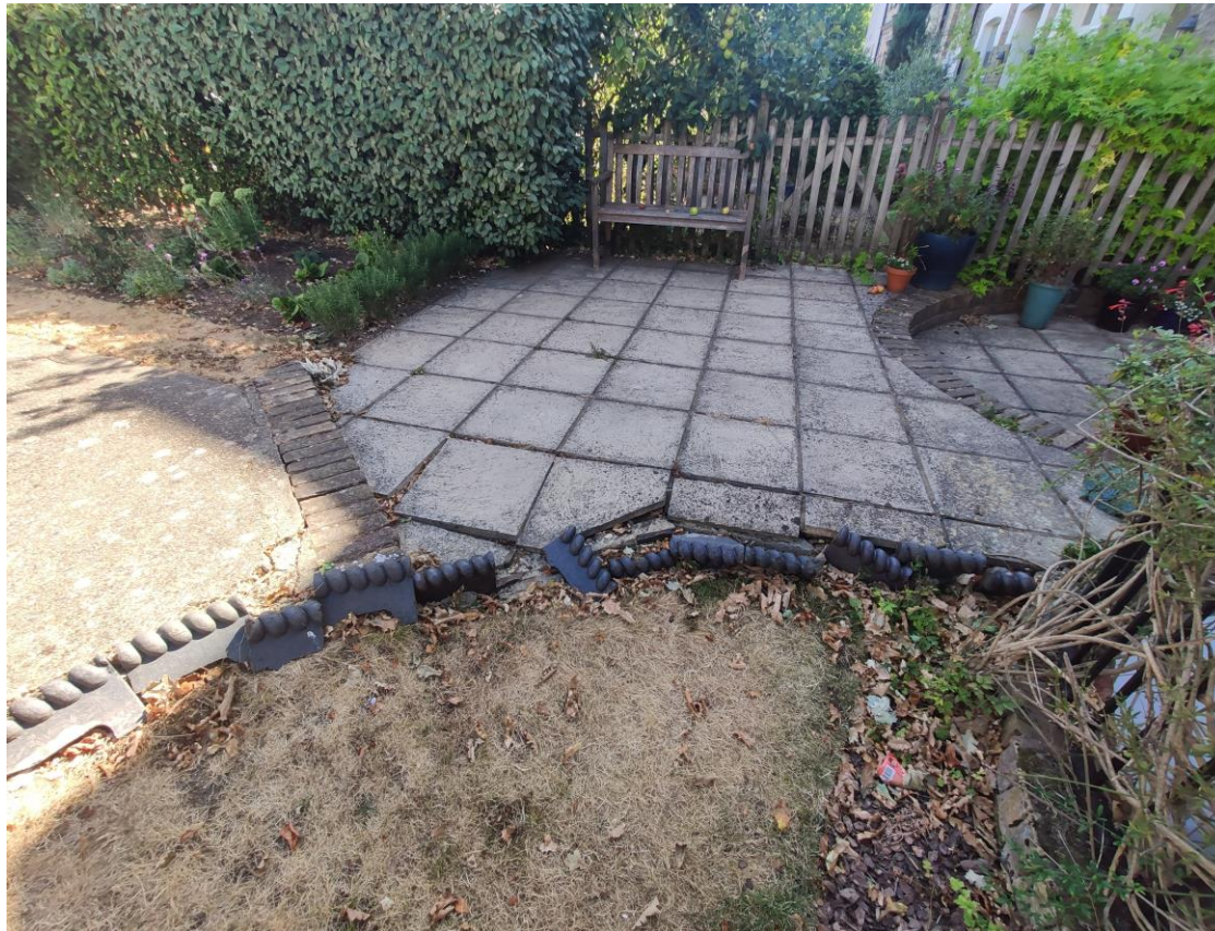
Photograph 4 showing damage to front path at 1 St. Martin's Terrace.
