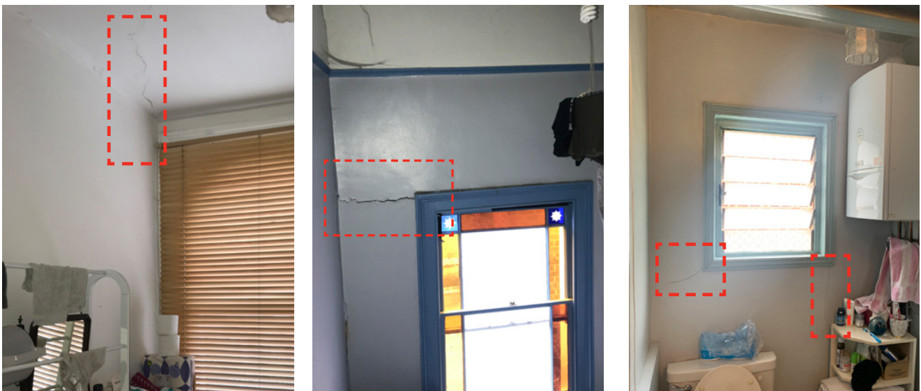
Fig 12 : Pictures of subsidence issues throughout the building
