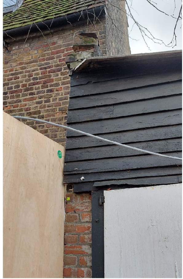
Loose Parapet at top of garage.
