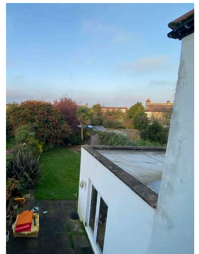
View of existing flat roof extension in poor condition
